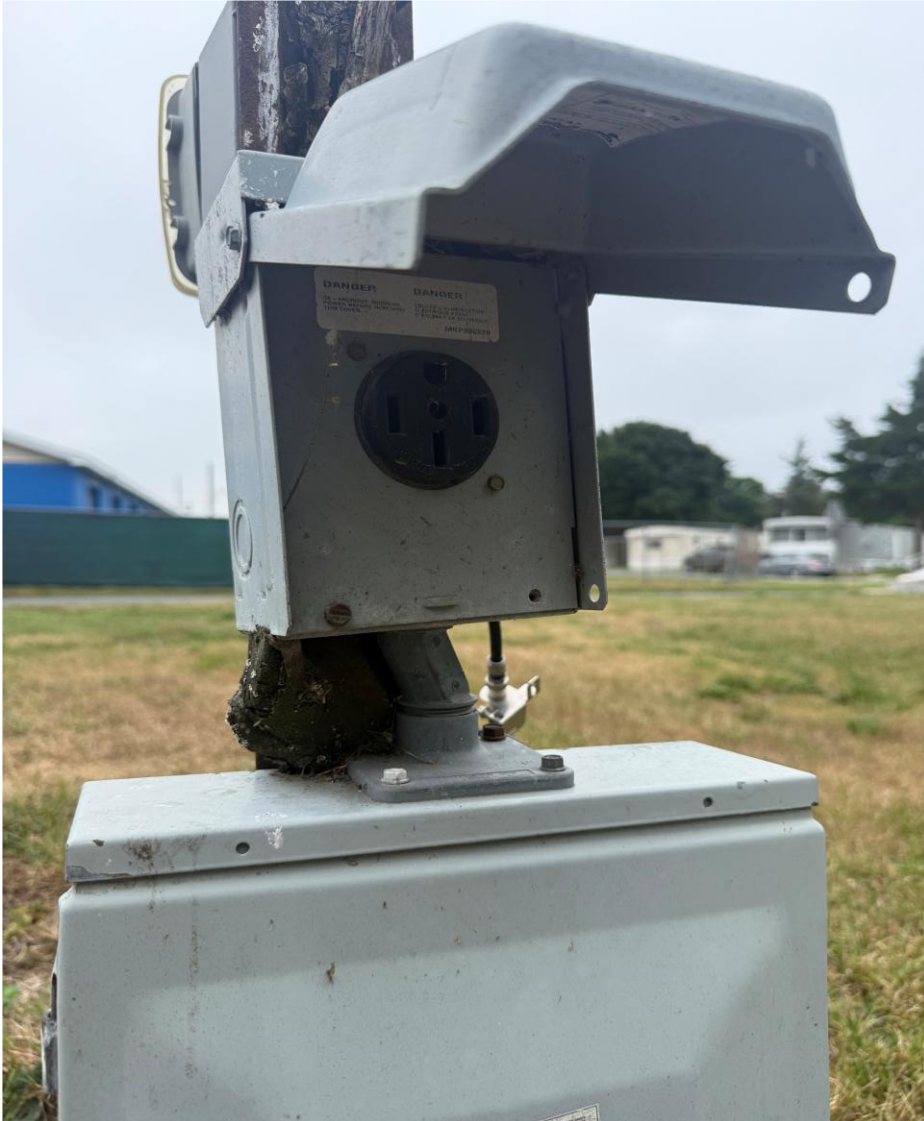
Electrical pedestal for RV site with a 50 amp hookup (Lot 142)
