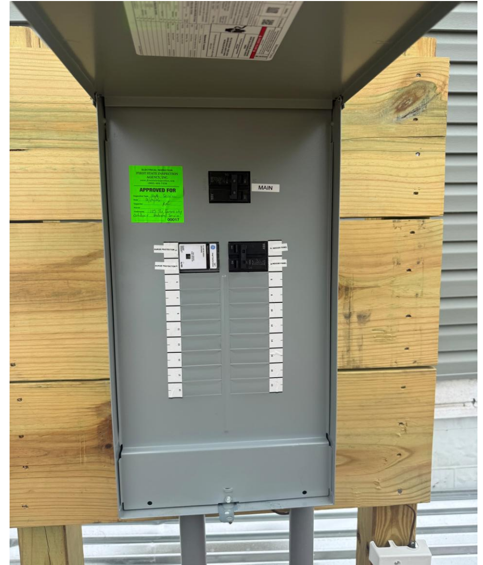
Electrical Pedestal for typical MH home site with a different mechanism for hooking up to electric
