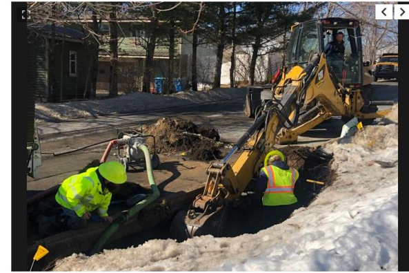
Grand Haven Department of Public Works employees work to fix a water main break on Howard Avenue in Grand Haven on Tuesday, March 2, 2021.
