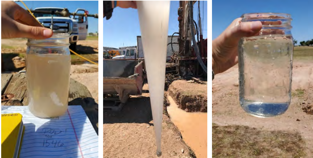
Figure 2-3: Progression of Well Development – Stantec will closely monitor development progress to track well performance and sand production.
