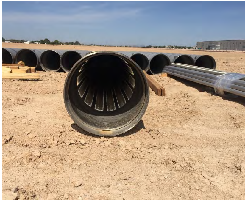
Figure 2-2: Well Casing and Sounding Tube Materials – Stantec will inspect all materials for conformance with the specifications.
