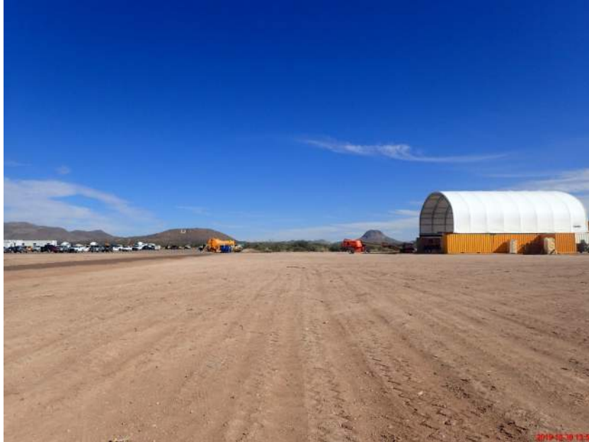
View from the northwest corner of the proposed project staging area looking east depicting U.S./Mexico border fence construction staging.
