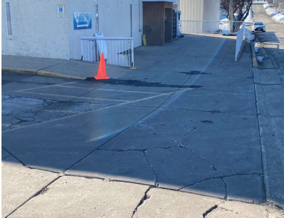
Photo 1: Concrete area west of SWCAP building. Asphalt patching was placed in an attempt to correct drainage issues.
