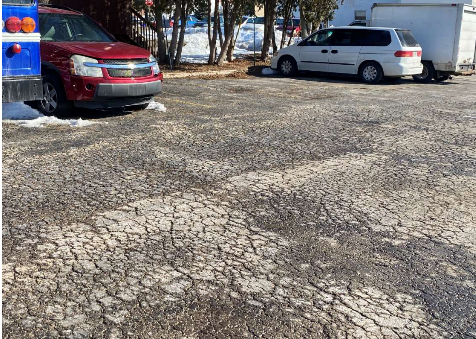
Photo 7: View of poor asphalt conditions in the west parking lot (east side of lot).
