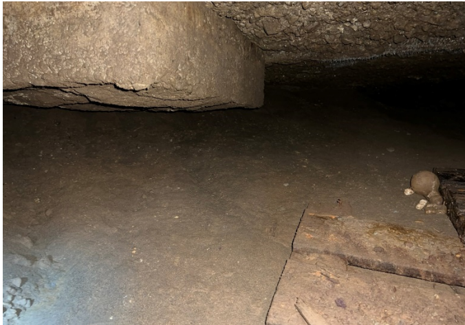
Figure 3: Void beneath column footing
