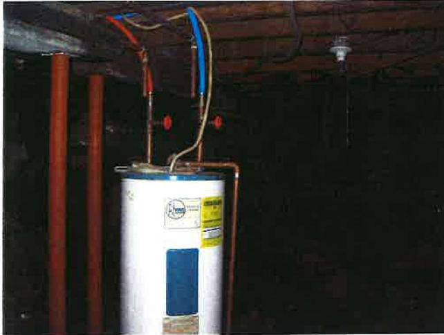
Water Heater in crawl space
