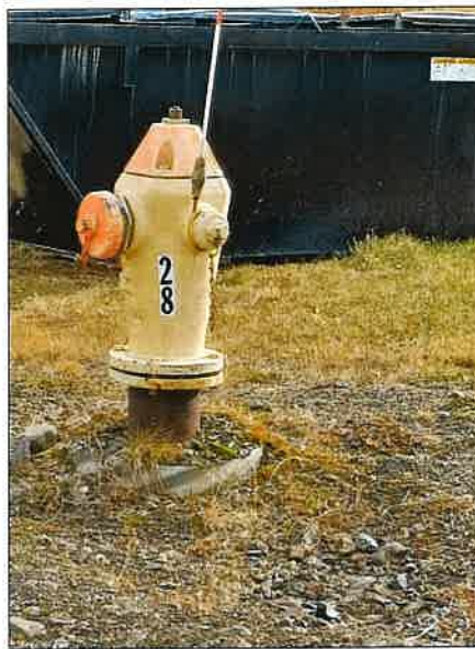
#25 Next to BBHA Office Building – Notice number on hydrant different then map.
