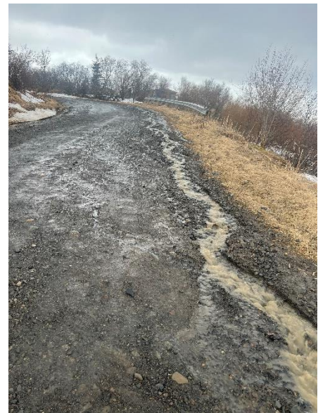
7 Road wash occurring at bottom of hill
