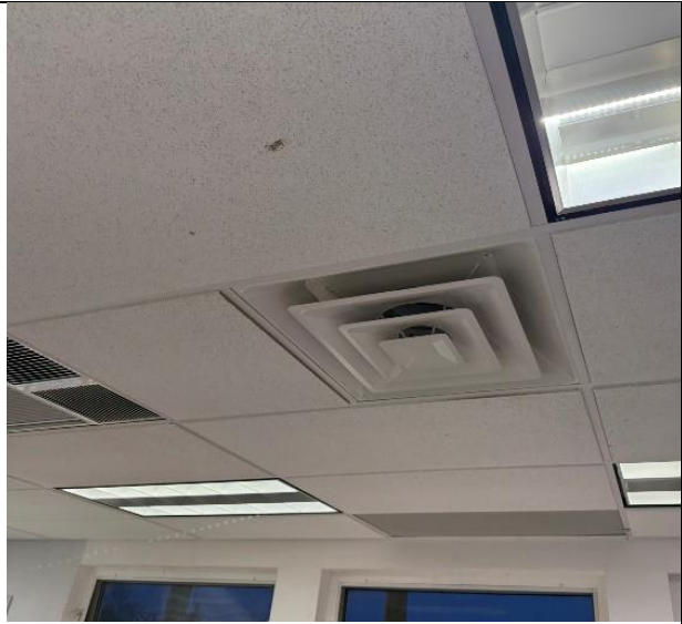
Forced Air heating
