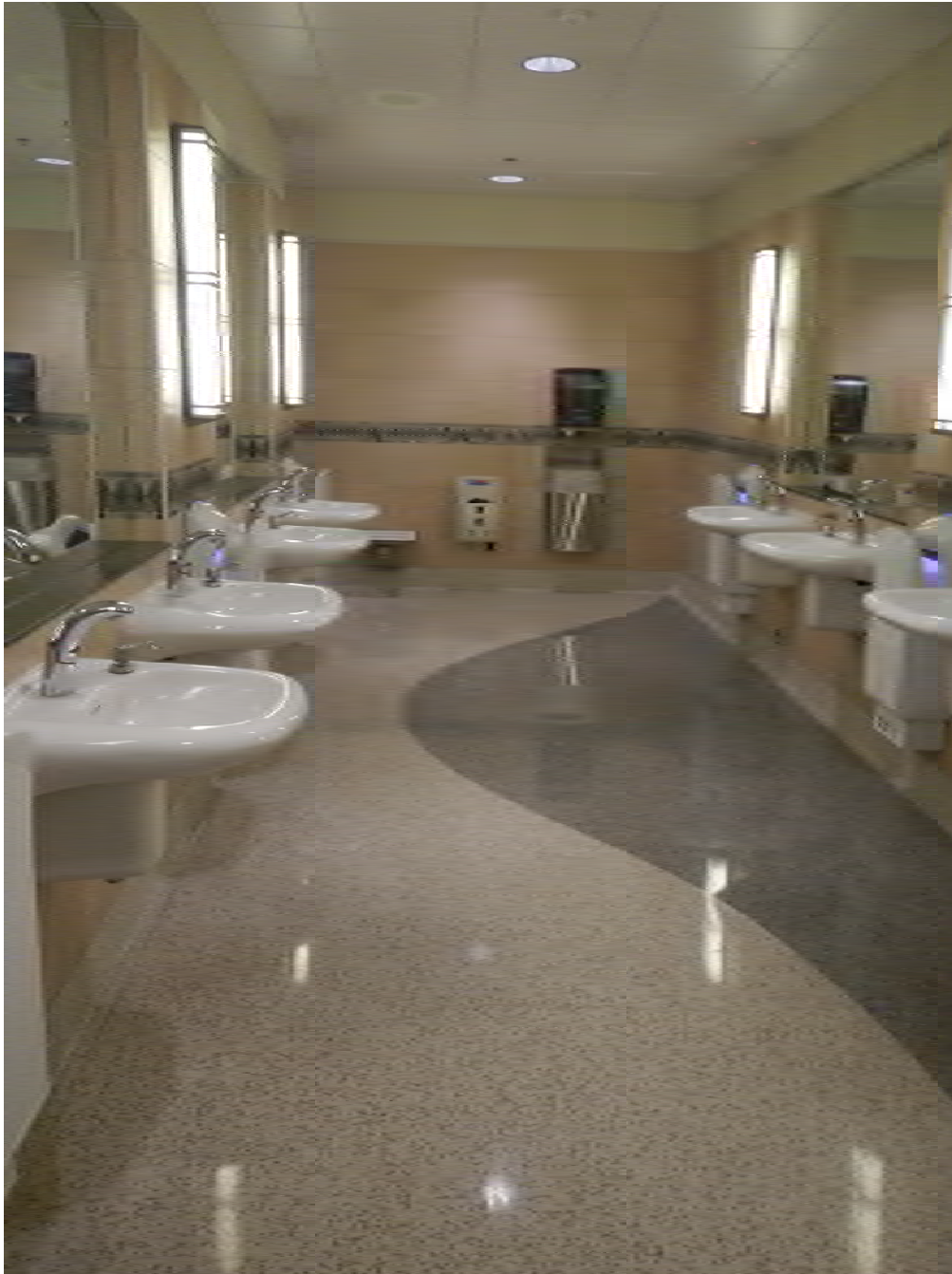
Figure 16 : Terminal restrooms offer both hand dryers and paper towel dispensers
