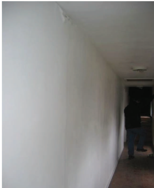
Photo No. 6: Corridor along south side of building at girder truss bearing.
