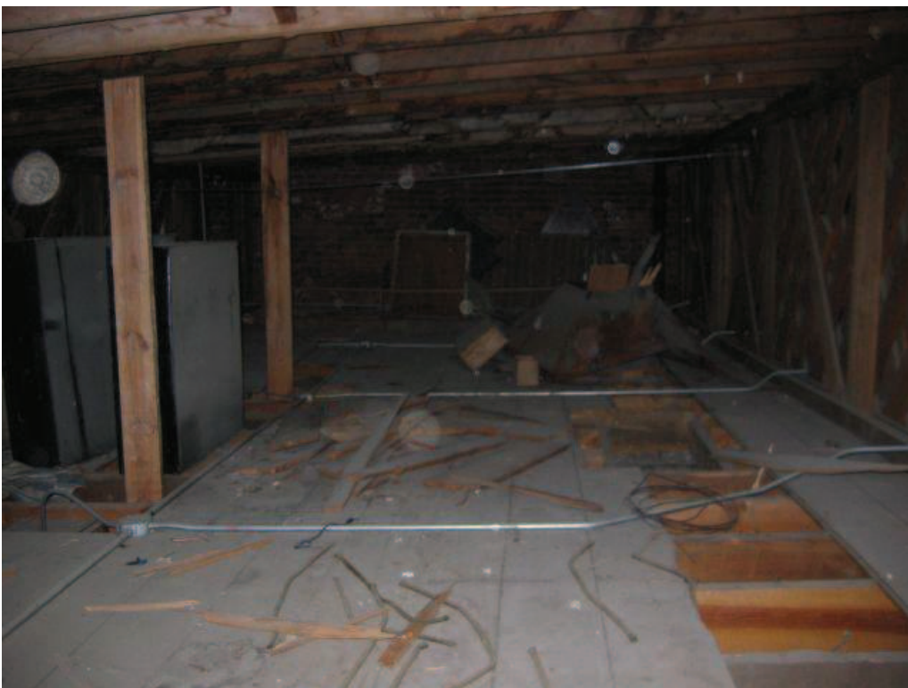
Photo No. 22: Typical ceiling and roof framing with floor planks on west side of subject girder truss.
