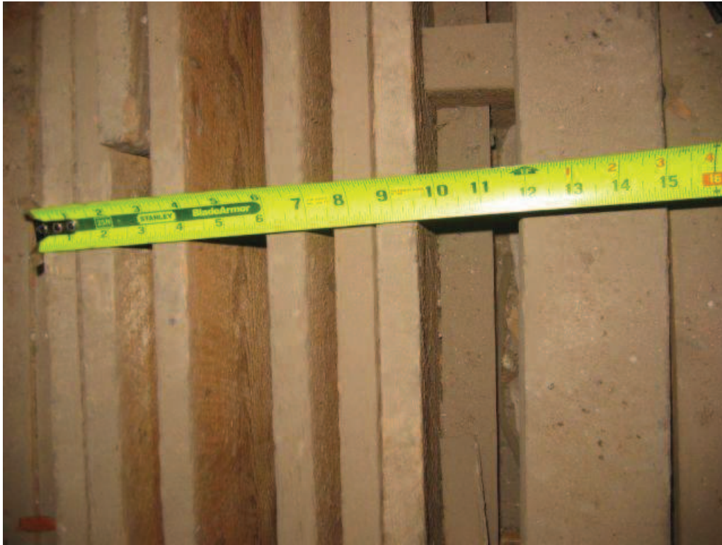
Photo No. 19: Spacing of bottom chord boards to allow for diagonal chord members.
