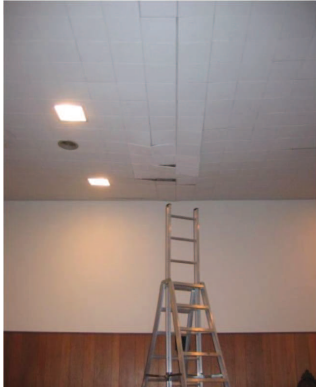
Photo No. 1: Displaced ceiling tile in auditorium at north end of girder truss.
