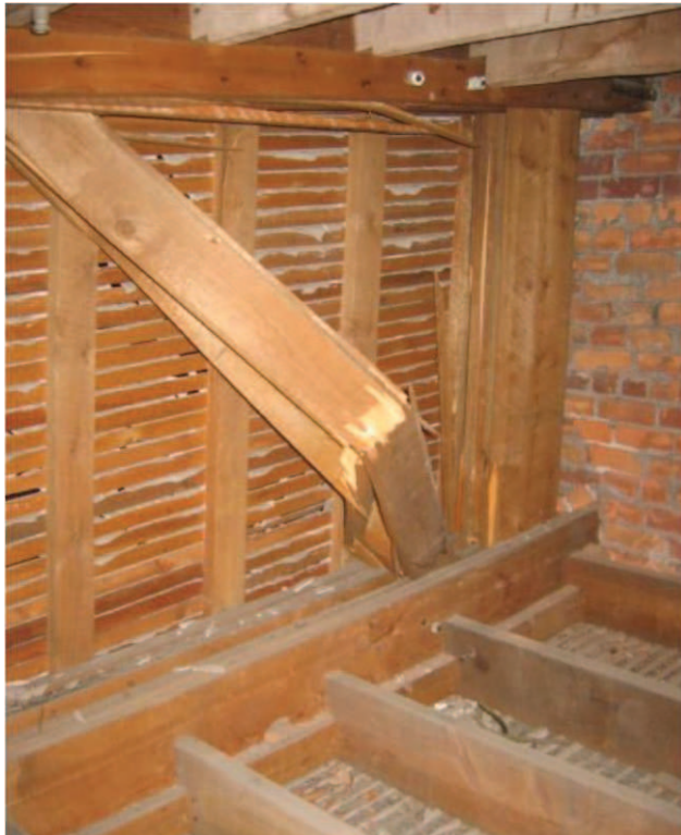
Photo No. 12: Breakage of diagonal chord member at north end of girder truss.
