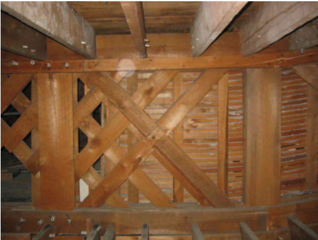
Photo No. 24: Interior panel of subject girder truss. View is at the north end, looking to the west.
