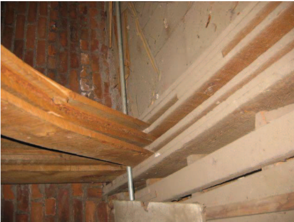
Photo No. 16: Breakage of the diagonal at south end of girder truss.
