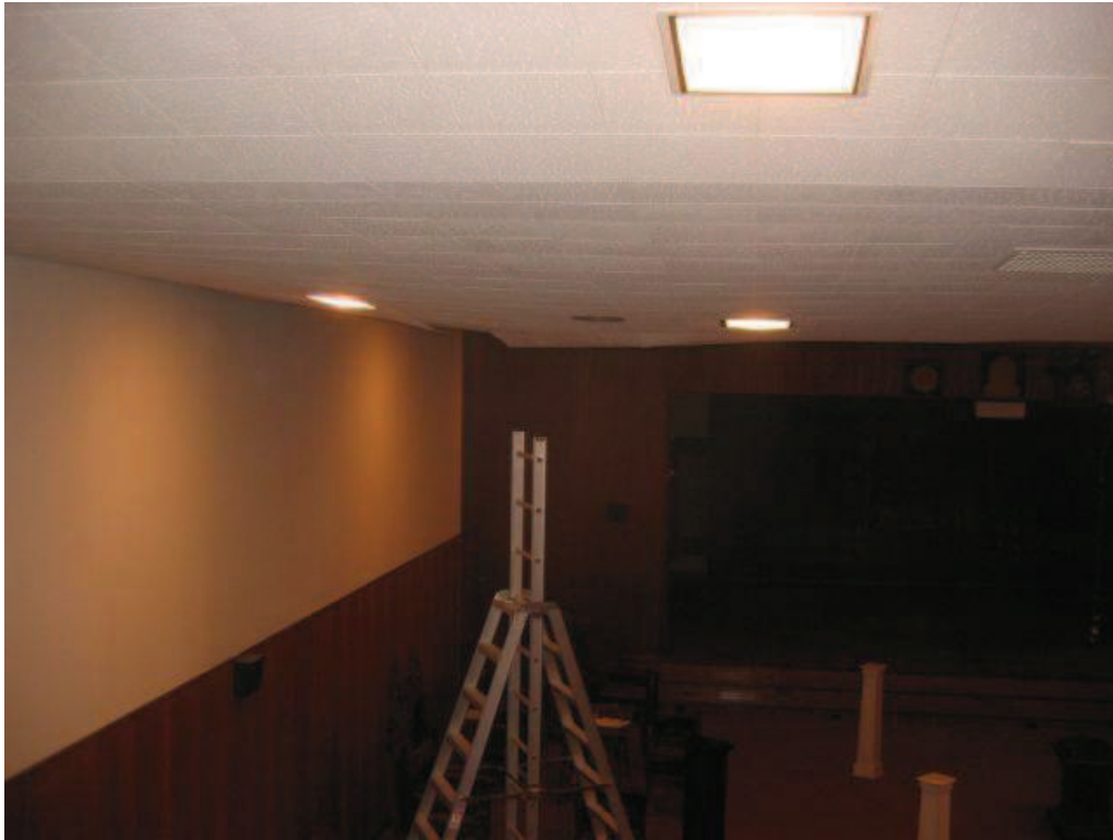
Photo No. 5: Deflection of ceiling tile at auditorium at north end of girder truss bearing.
