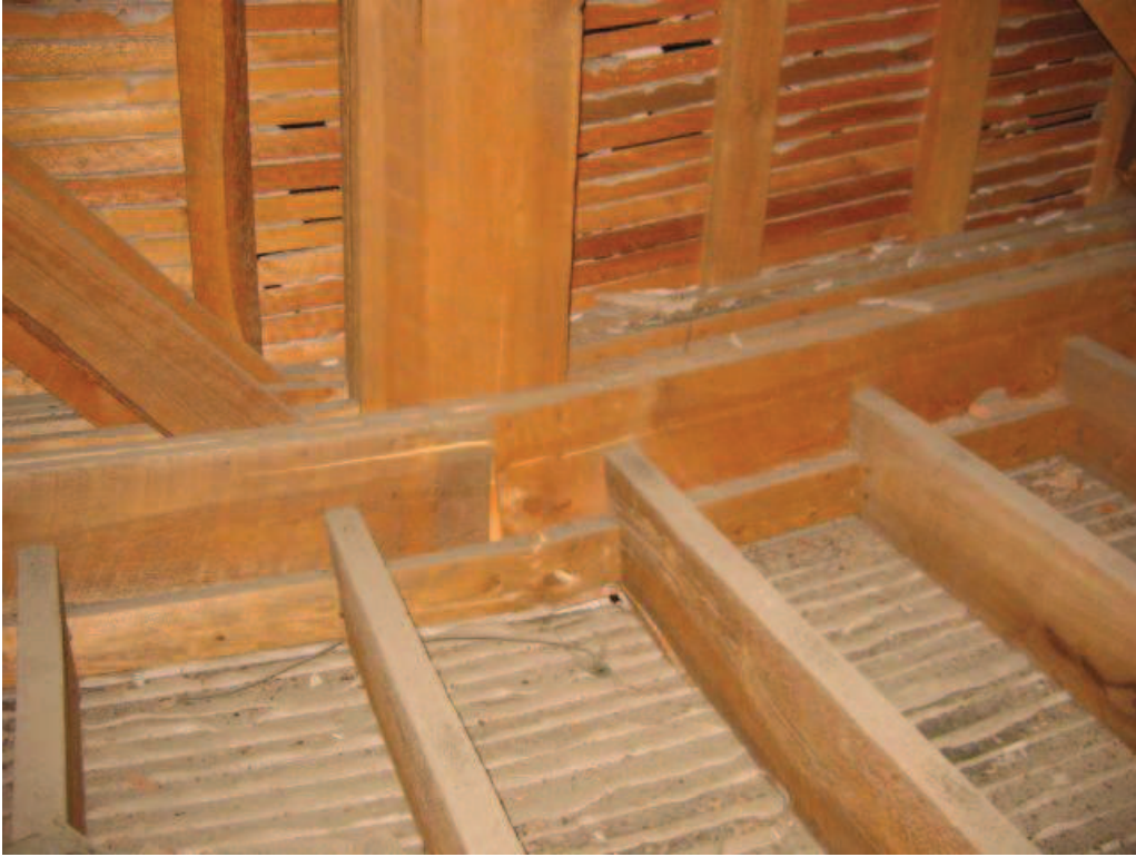
Photo No. 11: Breakage of the bottom chord boards at north end of girder truss.
