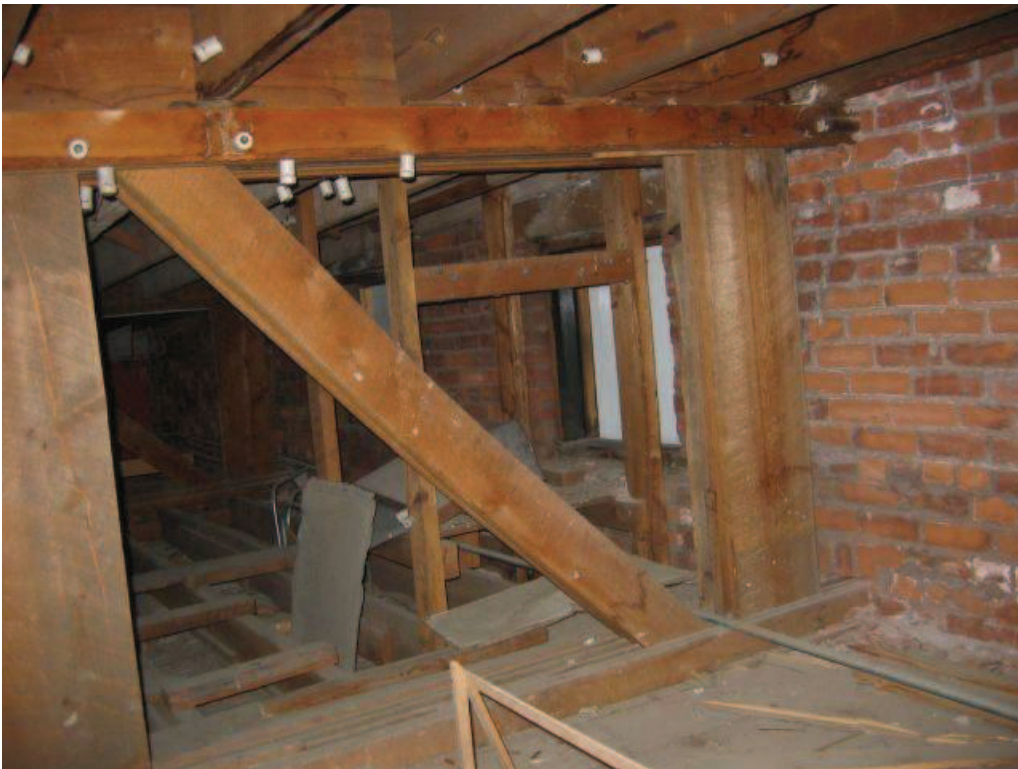
Photo No. 18: South end of girder truss, bearing point on brick wall.
