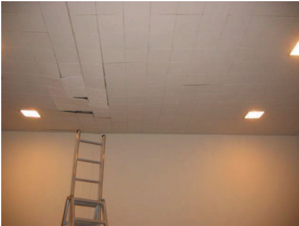
Photo No. 2: Displaced ceiling tile in auditorium at north end of girder truss.
