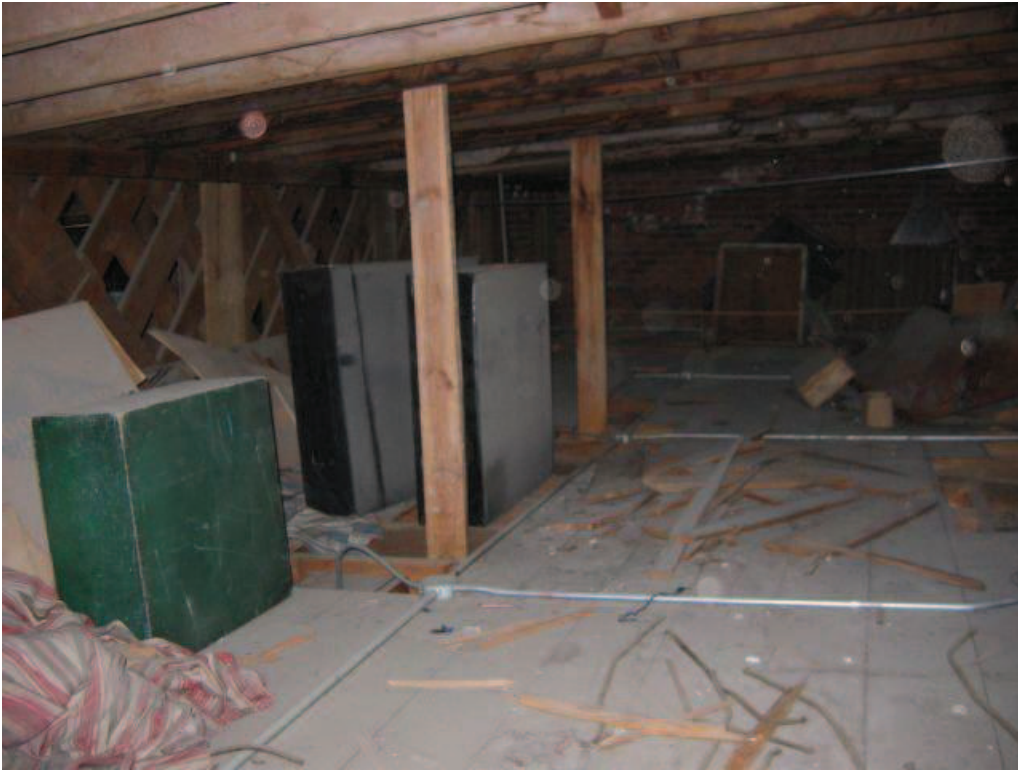
Photo No. 21: Typical ceiling and roof framing with floor planks on west side of subject girder truss.
