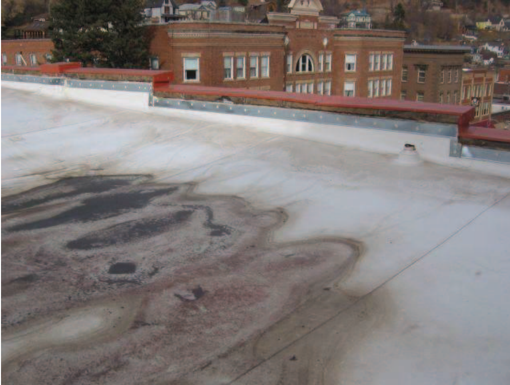
Photo No. 41: Significant drop / deflection at north end of subject truss. Note amount of sediment from long term water ponding.
