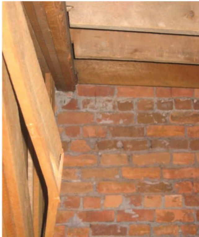
Photo No. 32: Girder truss to the east of subject girder truss. Breakage of the first panel diagonal at the north end.
