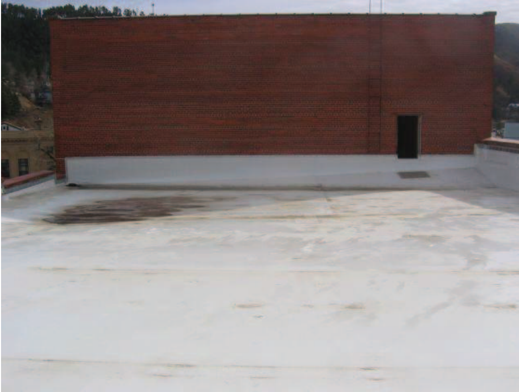
Photo No. 39: View of flyway wall at east end of lower roof.
