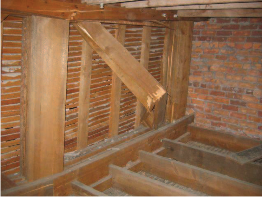
Photo No. 9: Overall view of broken girder truss members at north end of girder truss.
