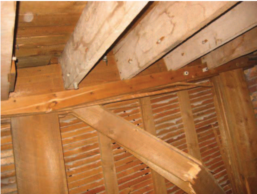
Photo No. 10: Breakage of the top chord boards at the north end of the girder truss.
