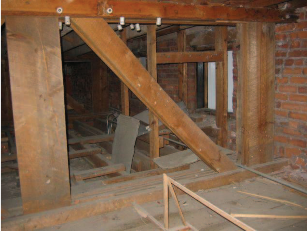
Photo No. 17: Breakage of the vertical chord member at south end of girder truss.
