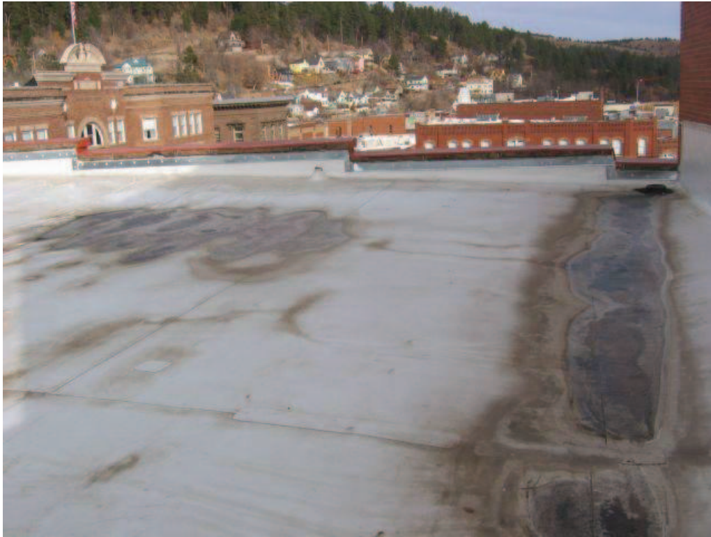
Photo No. 33: North parapet at drain inlet. Note sediment from long term water ponding.
