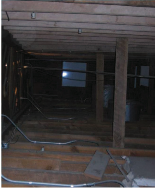
Photo No. 23: Typical ceiling and roof framing on east side of subject girder truss.
