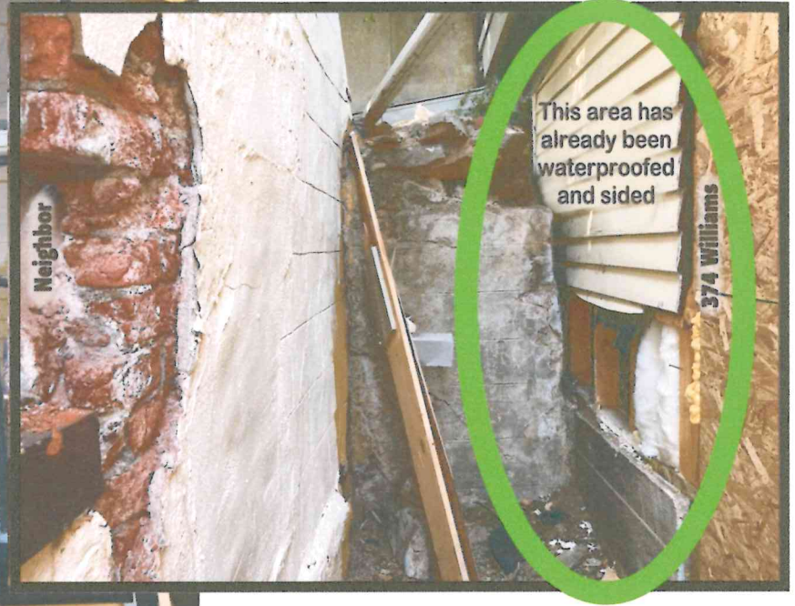
Visible water damage on neighboring property
