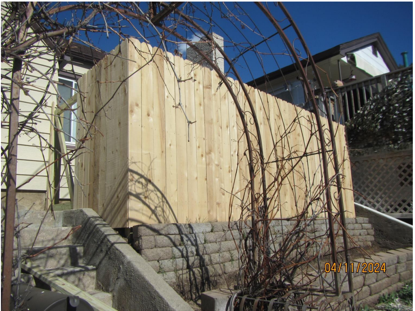
Fence covering the front window on right front side of structure.
