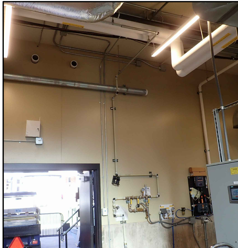
5 EQUIPMENT MOUNTING SPACE PHOTO
