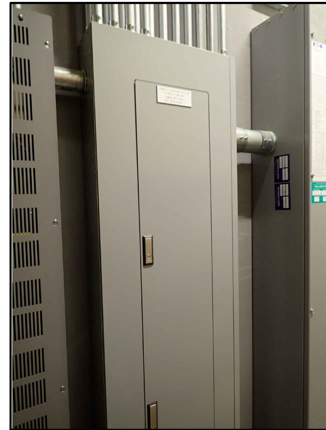
3 POWER PANEL PHOTO
