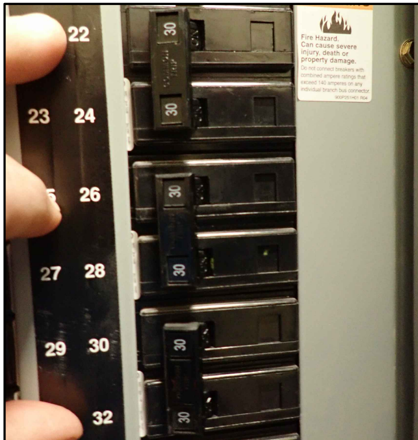
4 ELECTRICAL BREAKERS PHOTO
