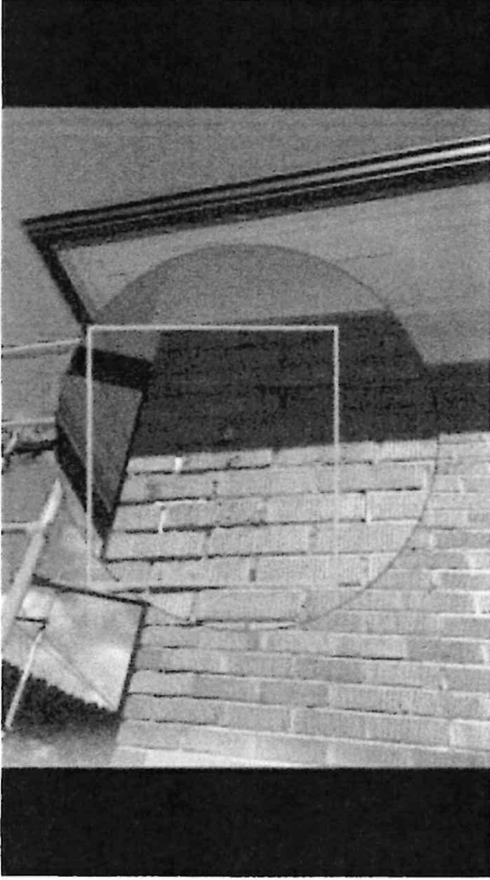
Area where brick needs restoration
