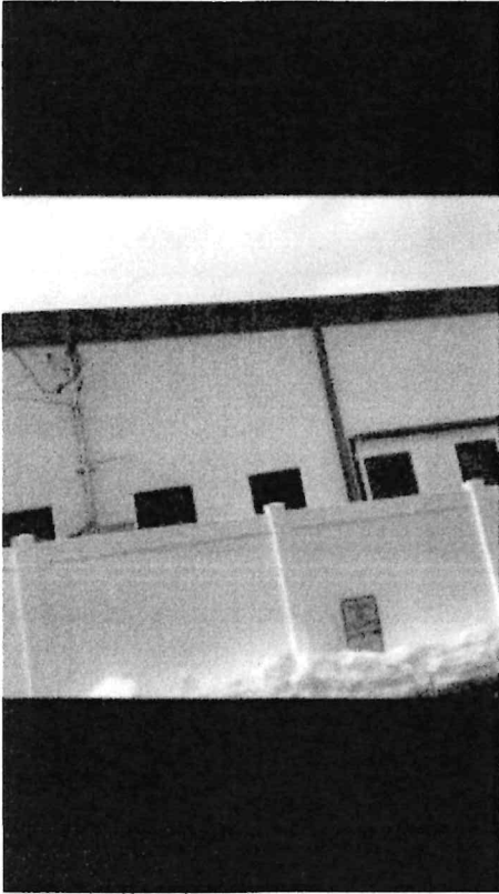
Back Stucco is peeling in areas and needs to be removed. Caulking and sealing masonry.
