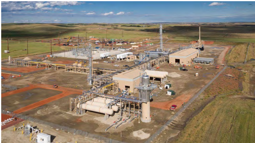
The Bear Creek natural gas processing plant in Dunn County. Image Credit: The Dickinson Press
