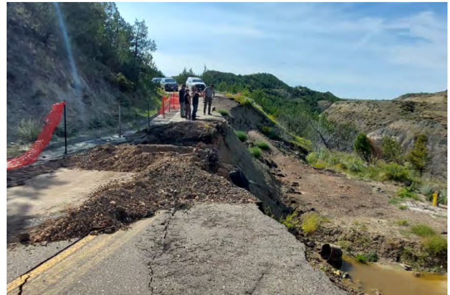
Part of the Scenic Drive Loop in the Theodore Roosevelt National Park South Unit collapsed in 2019. Crews have been working since 2022 to repair the six-mile stretch of road. Image Credit: Bismarck Tribune
