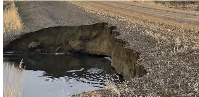
A washed-out section of 92 nd Avenue in Dunn County.
