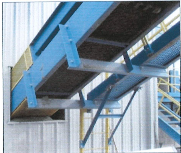
Figure 9. Shredder conveyor opening.
