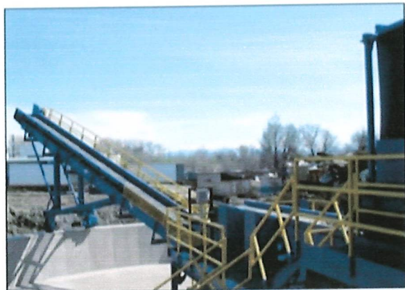
Figure 2. Shredder system conveyor.
