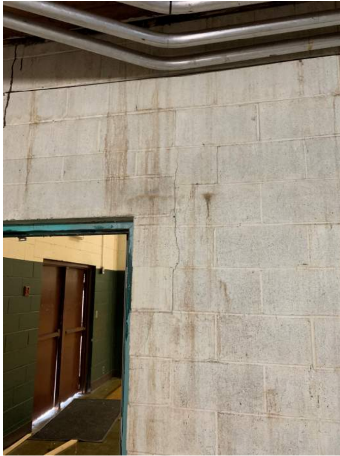
Photograph N: Cracks on Storage Room #1 CMU Wall (Looking South)
