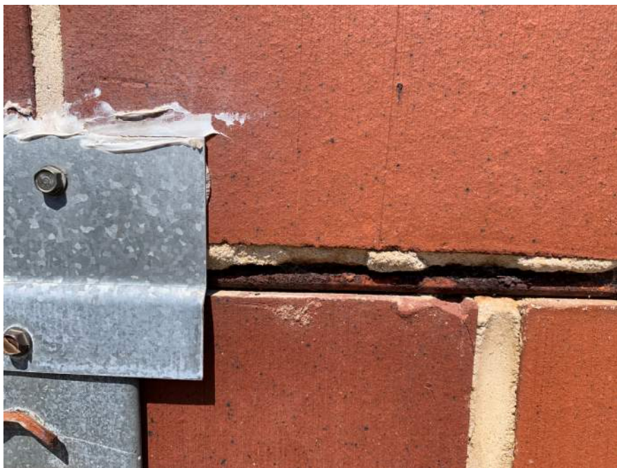
Photograph P: Rusted Steel Shelf Angle (Looking West)
