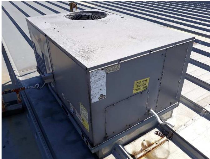
Upper Office Area Rooftop Unit
