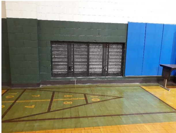
Gymnasium Ventilation Intake Louvers
