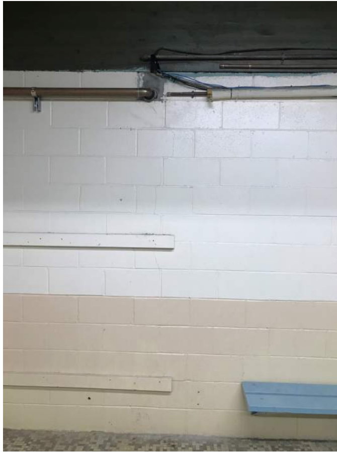
Photograph C: Cracks on Building A Men's Restroom CMU Wall #1
