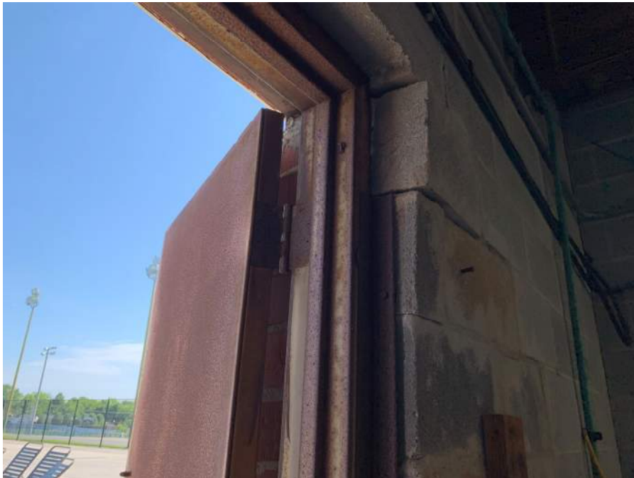
Photograph H: Building A Rusted Door Frame
