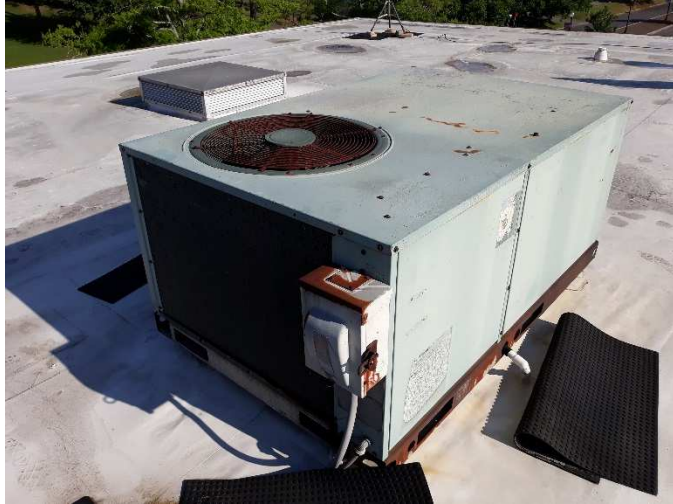
Original Multipurpose Rooftop Unit - Abandoned
