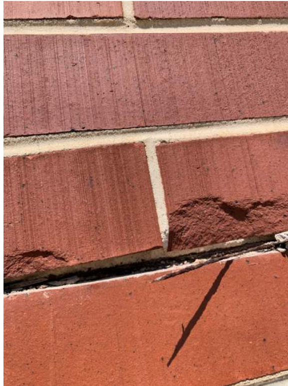
Photograph Q: Rusted Steel Wire Reinforcing (Looking North)
