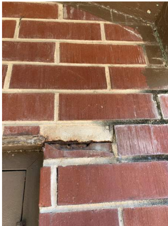
Photograph R: Cracks on Building B Brick Veneer (Looking North)
