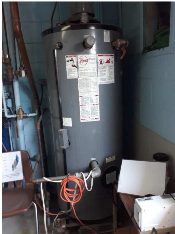
Pool Water Heater for Showers
