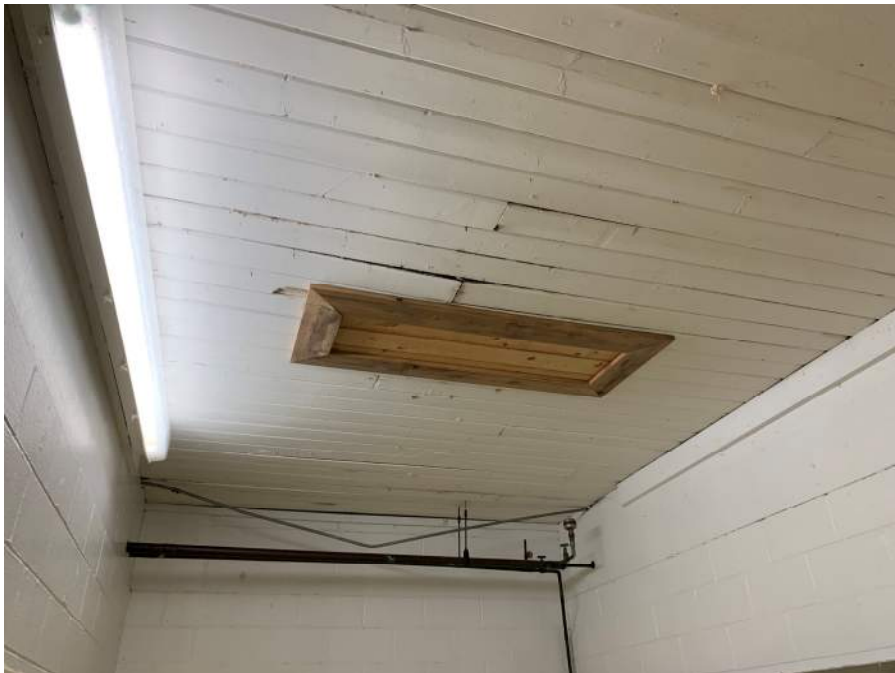
Photograph F: Cracks on Building A Men's Restroom Timber Decking
