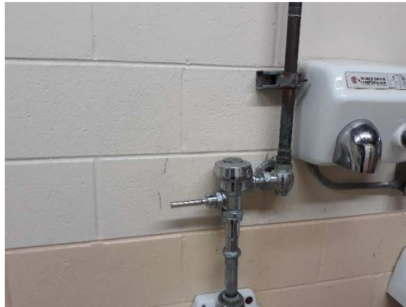
Locker Room Piping indicating corrosion
