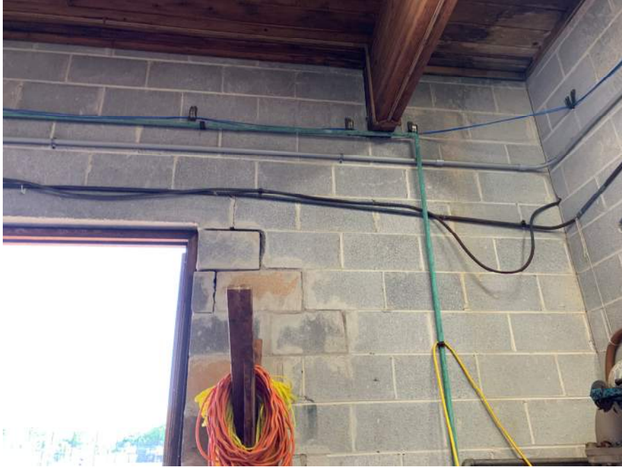
Photograph E: Cracks on Building A Pool Mechanical Area (Looking North)
