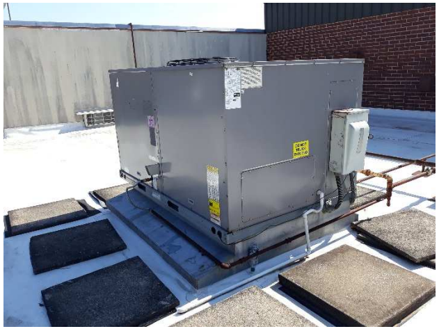
Rooftop Unit for Original Building
