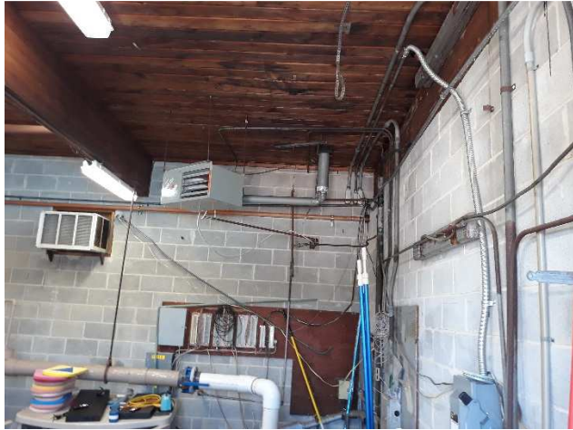
Pool Equipment Area – Window Unit from Storage
