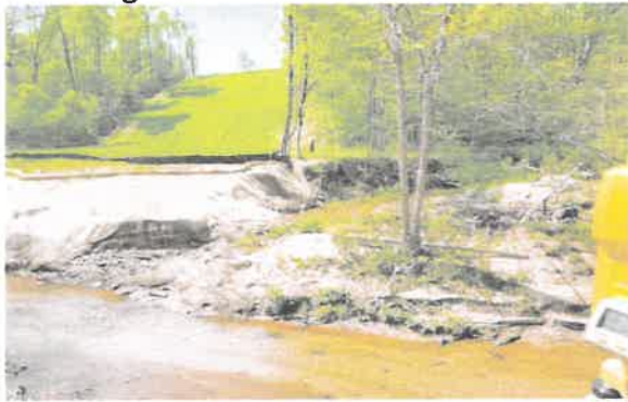
Blow out after gas line install due to Hurricane
