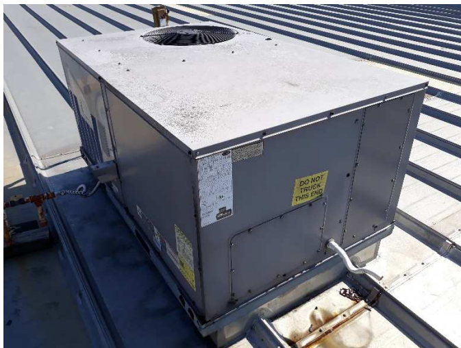
Upper Office Area Rooftop Unit
