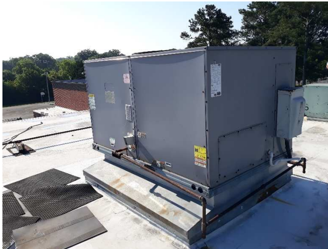
Replacement Multipurpose Rooftop Unit
