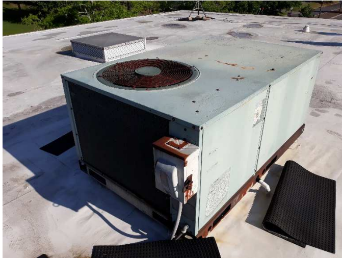
Original Multipurpose Rooftop Unit - Abandoned
