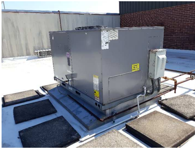
Rooftop Unit for Original Building
