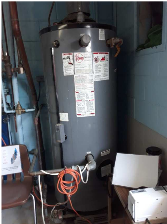
Pool Water Heater for Showers
