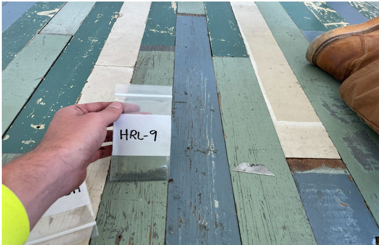
Plate 13: Laboratory analyses detected 1.5% lead within the blue floor paint within sample HRL-9 collected from the interior of the structure.
