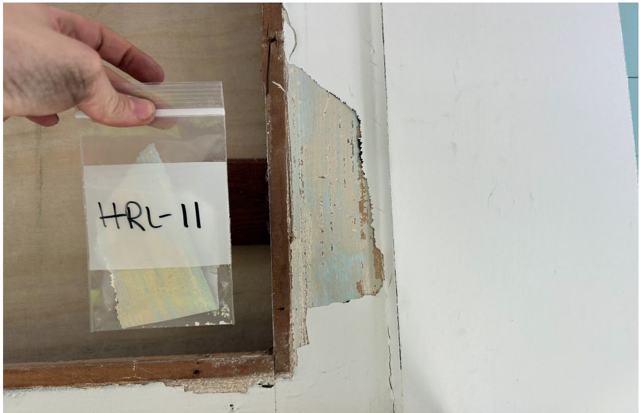
Plate 15: Laboratory analyses detected 1.4% lead within the white fireplace paint within sample HRL-11 collected from the interior of the structure.
