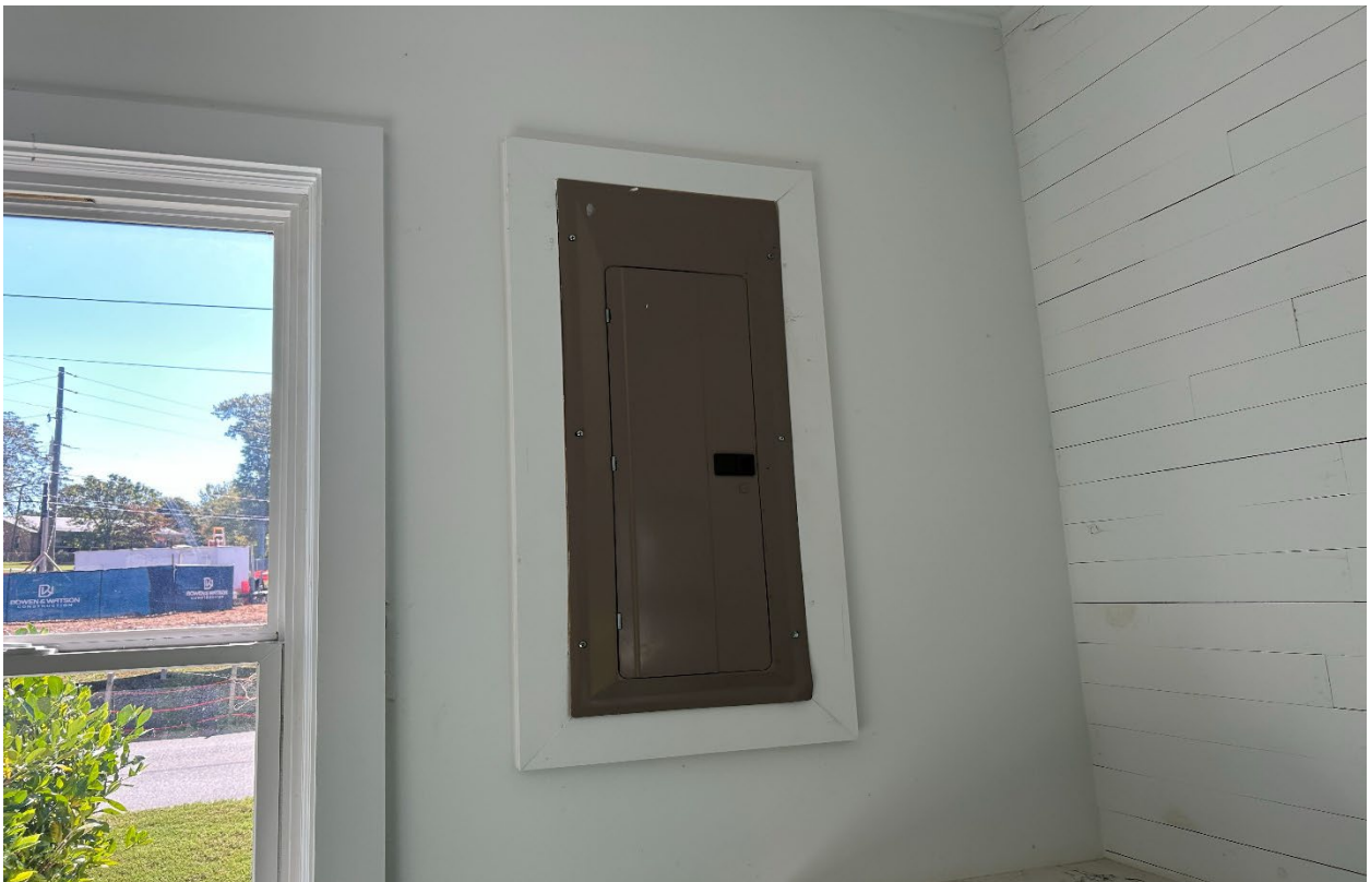
Plate 6. Photograph of typical electrical panel containing assumed asbestos containing insulation materials at the structure at the subject property.
