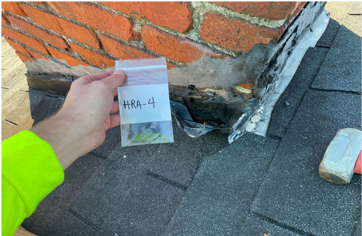
Plate 7. Laboratory analyses detected 10% chrysotile asbestos minerals within the black penetration flashing and tar within samples HRA-3 and HRA-4 collected from the chimney of the subject property structure. All black penetration tar at the subject property should be considered asbestos containing material.
