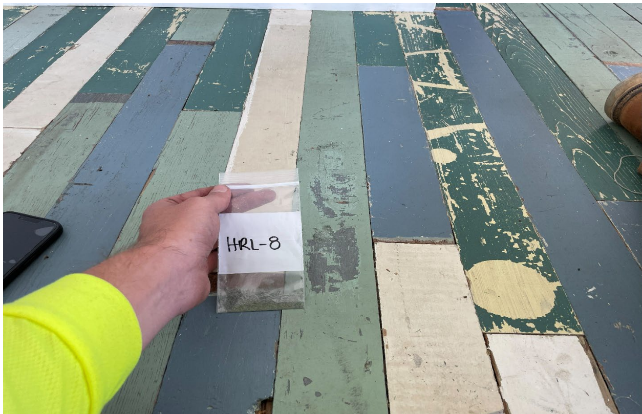
Plate 12: Laboratory analyses detected 0.69% lead within the light green floor paint within sample HRL-8 collected from the interior of the structure.
