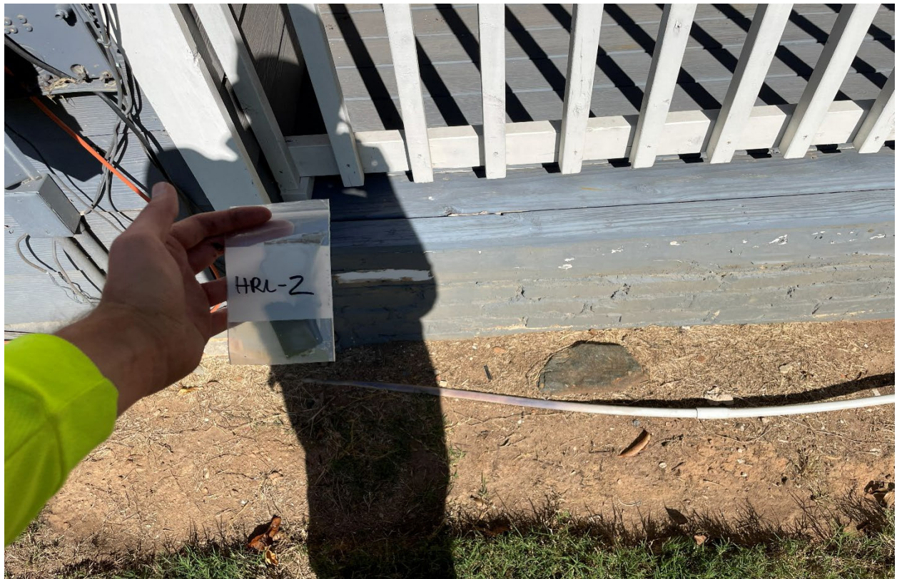
Plate 9: Laboratory analyses detected 0.052% lead within the blue paint within sample HRL-2 collected from the exterior of the structure.
