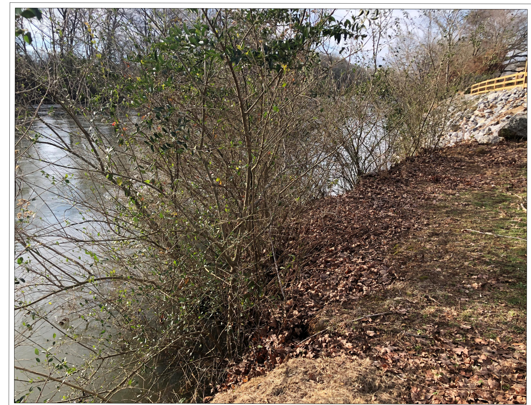
PICTURE "4" RIVER BANK ERODING
