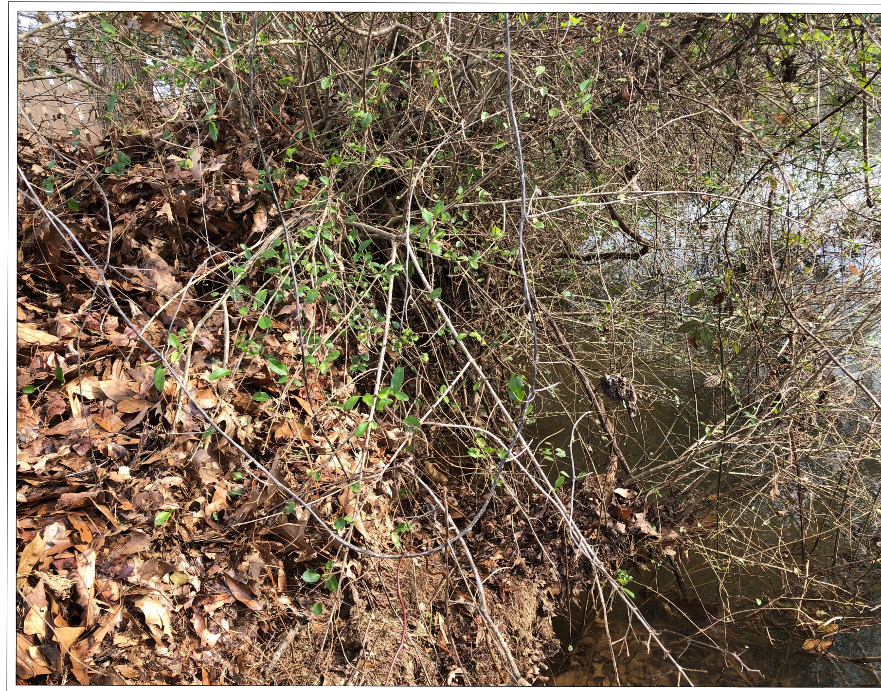
PICTURE "3" RIVER BANK ERODING
