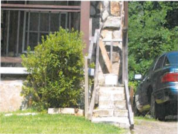
These front steps need to be replaced.
