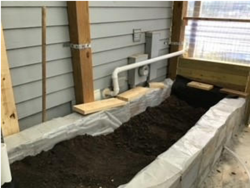
Electric meter is inside the greenhouse.
