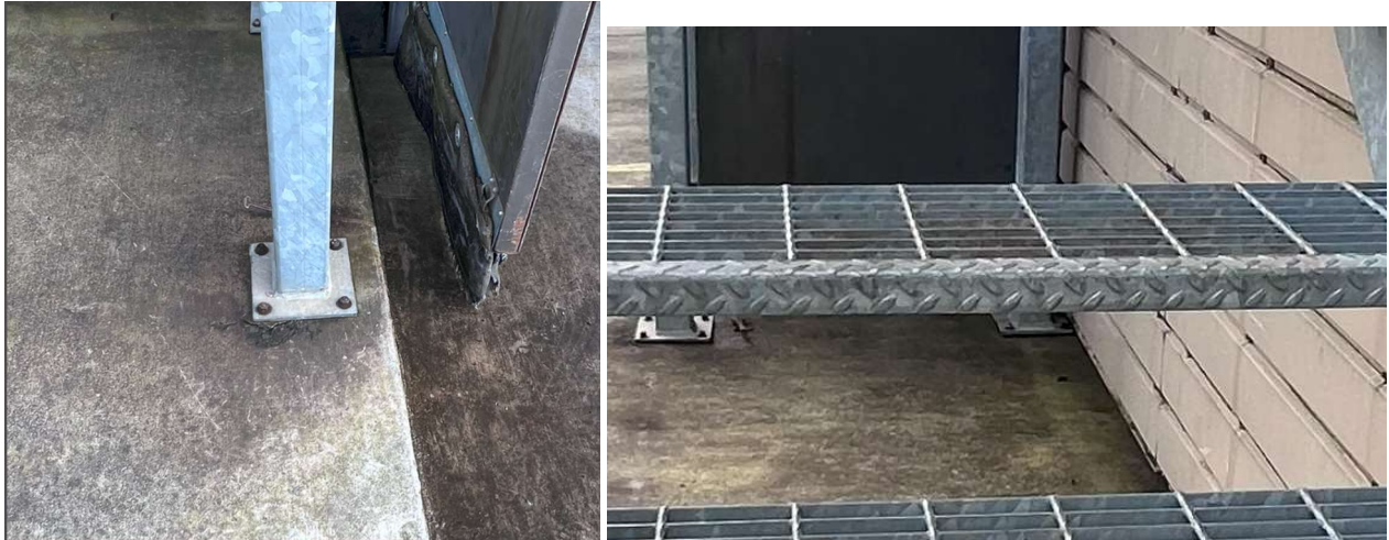
Rusting at Exterior Stair Column Baseplate/Rusting at Exterior Stair Grate Treads
