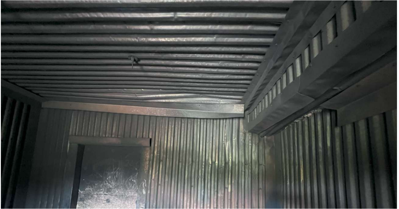
Burn Room #2 Warped Ceiling Panels & Trim
