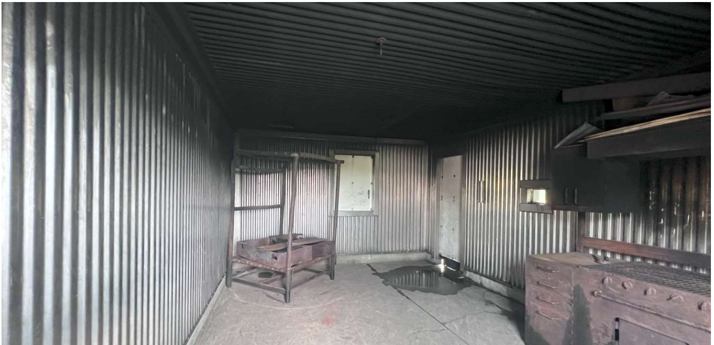
Annex Burn Room w/ Minor Warped Ceiling Panels
