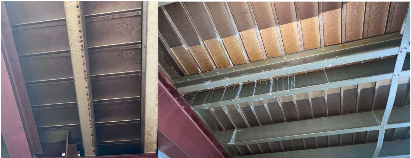
Corrosion/Rusting of Light Gauge Joists Below 2 nd Floor Concrete Deck
