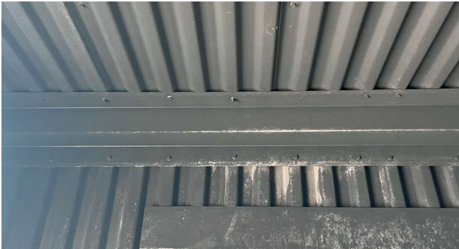
Backed out & Missing Ceiling Trim Screws
