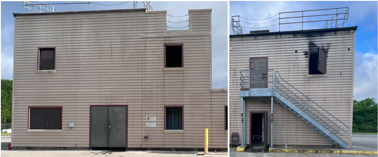
Rust Marks Along Screw Lines at Exterior Wall Panels/Soot Buildup Adjacent to 2 nd Floor Burn Room Door
