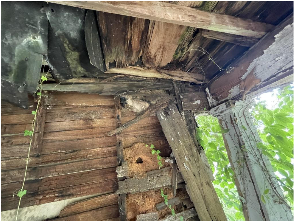
North wall of porch. Water Damage.
