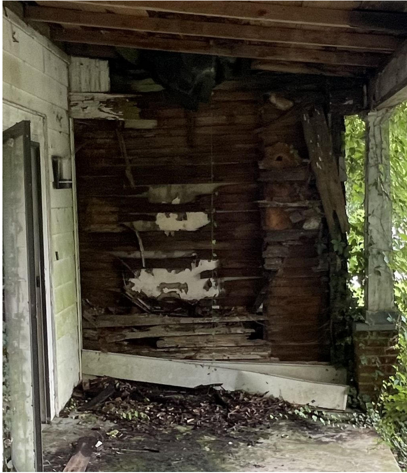
North wall of porch. Water Damage.
