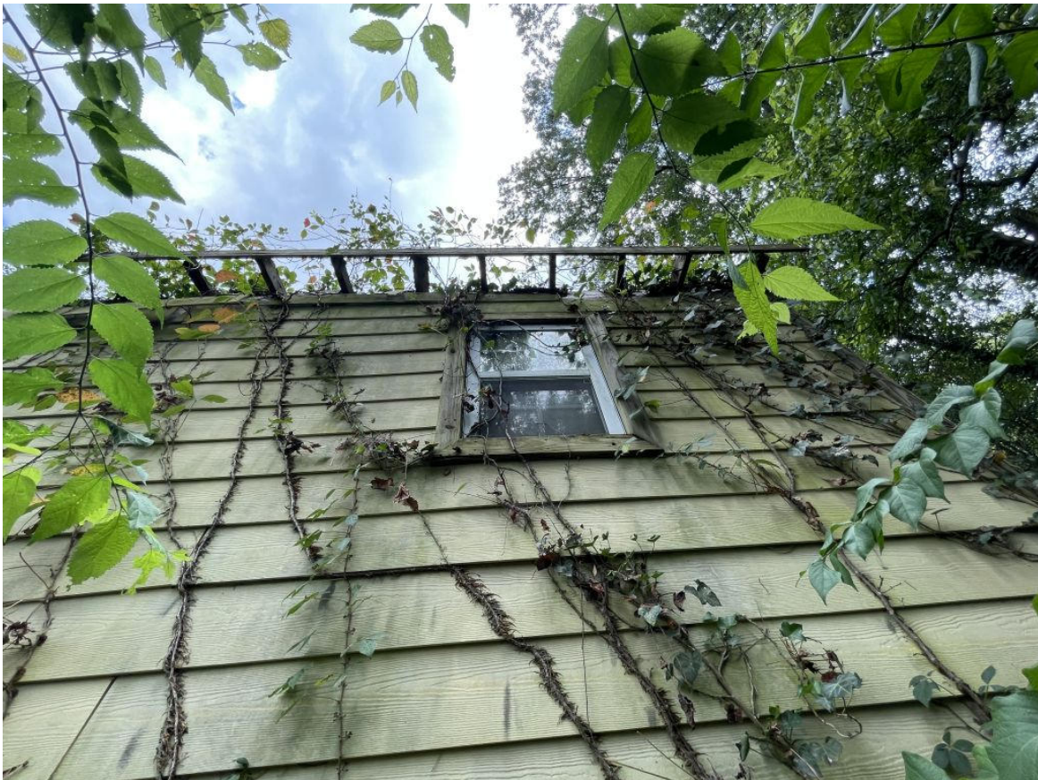
View to rear of home from SW corner. Roof missing on addition.
