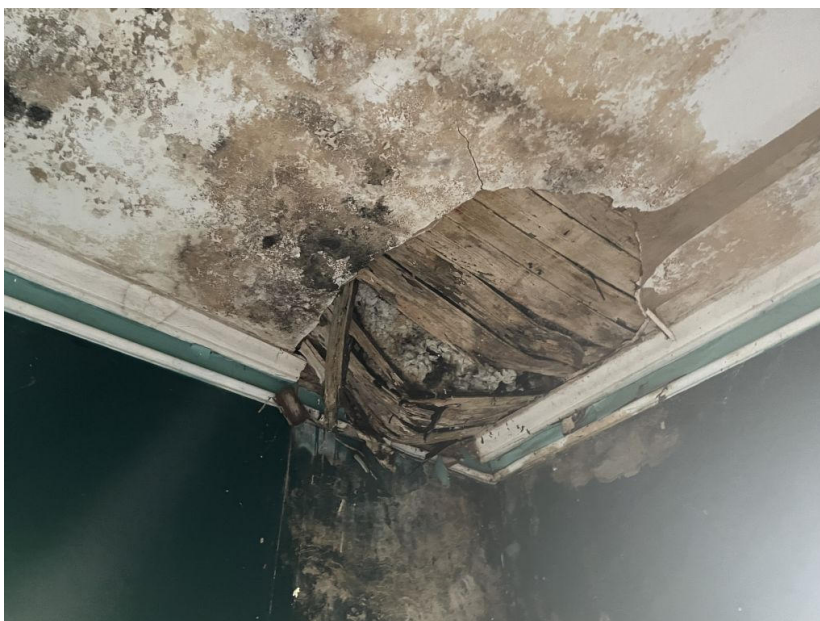
Foyer- Front Center Room at front door.. Rotted ceiling above rotted floor from water damage
