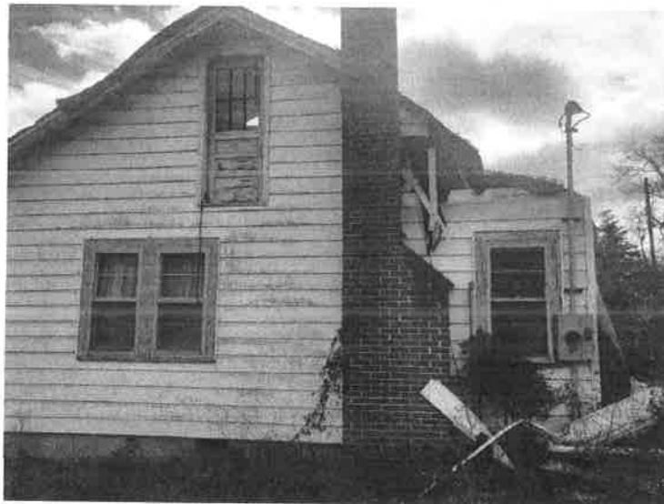
Damage to Front of the House
