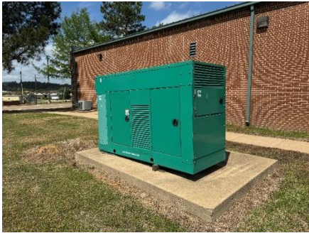
F: Natural Gas Generator
