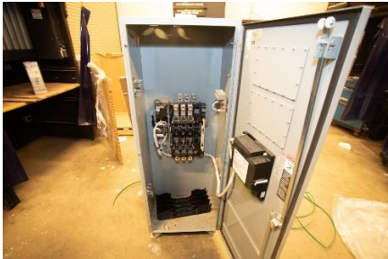
G: Electrical Transfer Switch
