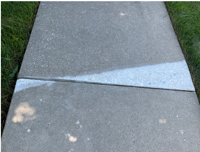
Sample Repair Photo: Defect 236 was repaired on 08/09/2024 at 21401 Abbey Ln at 11:06 AM
