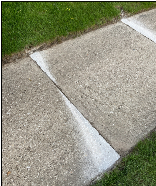
Sample Repair Photo: Defect 310 was repaired on 05/05/2025 at 1710 Arbor Ln at 5:39 PM
