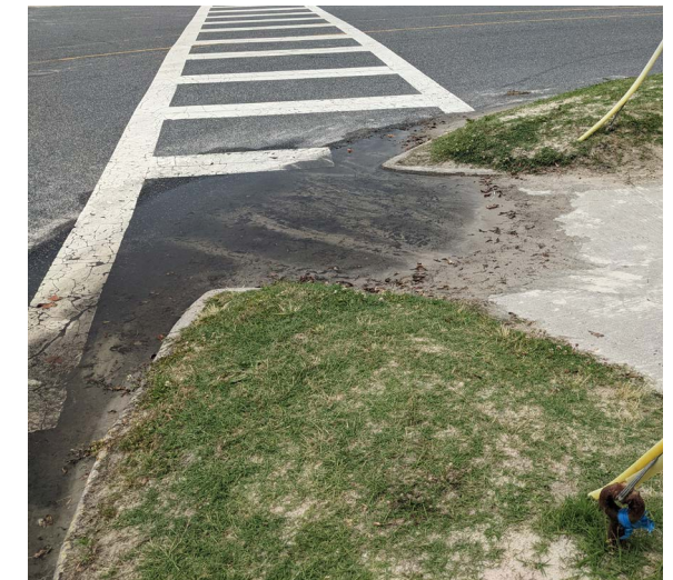
Storm water at a Mason Ave. crosswalk.
