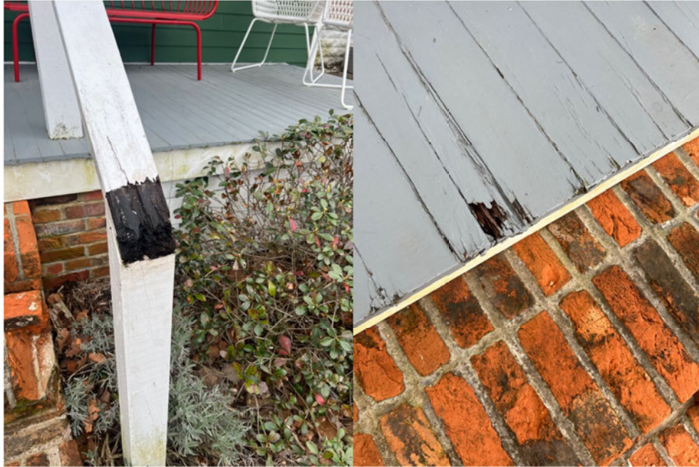
Current Photos of rotting temporary railing, porch decking and deteriorating brick steps.
