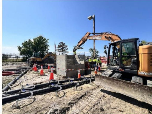
Mason Ave. Lift Station
