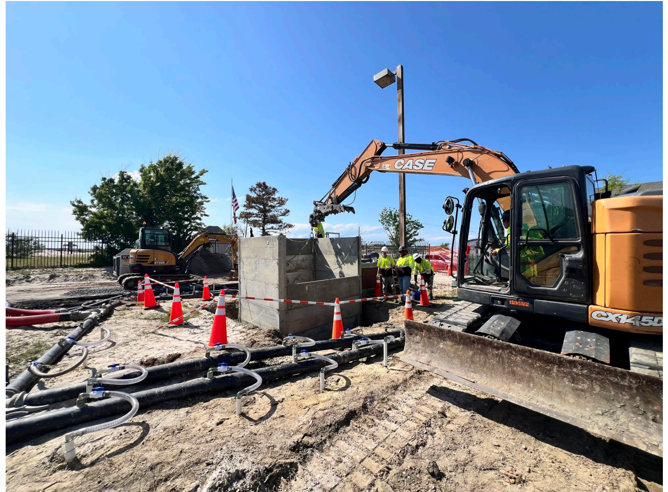
Mason Ave. Lift Station
