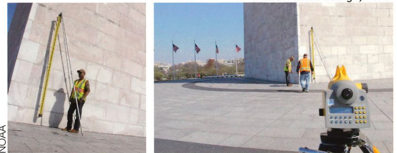
Assessing earthquake damage, 2012
