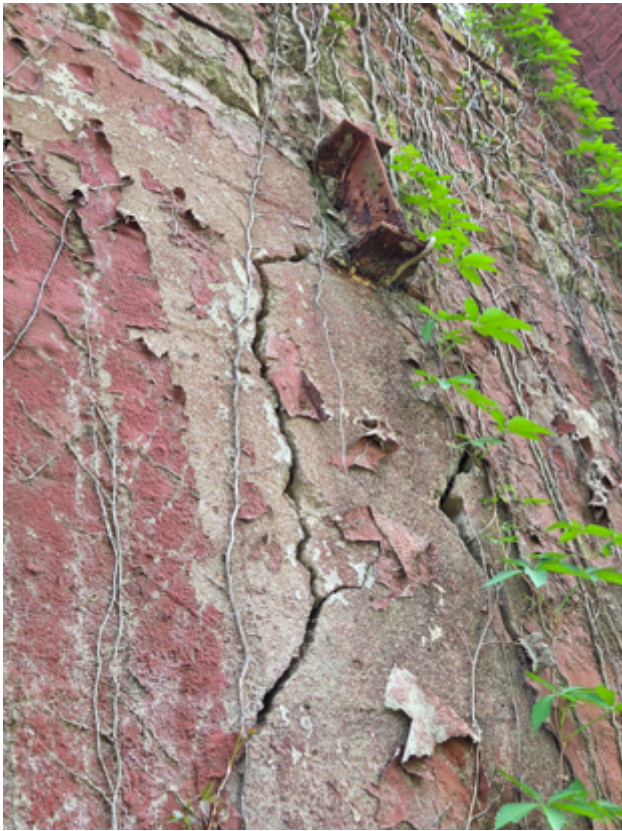
Cracking in Rear Wall
