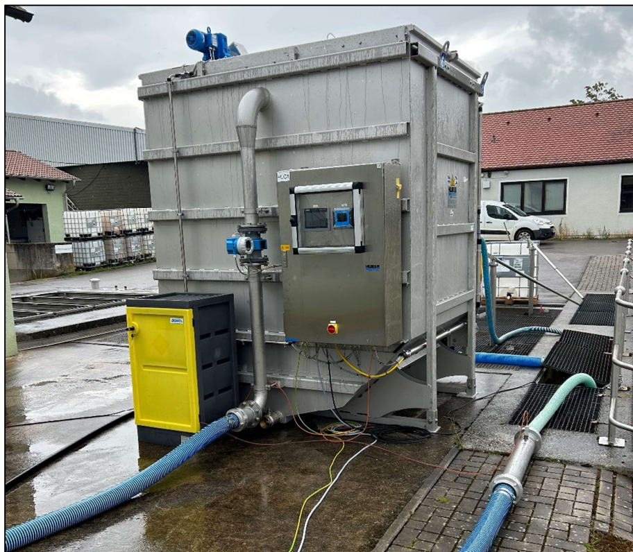
Chemical Dosing Cabinet; Static Mixer
