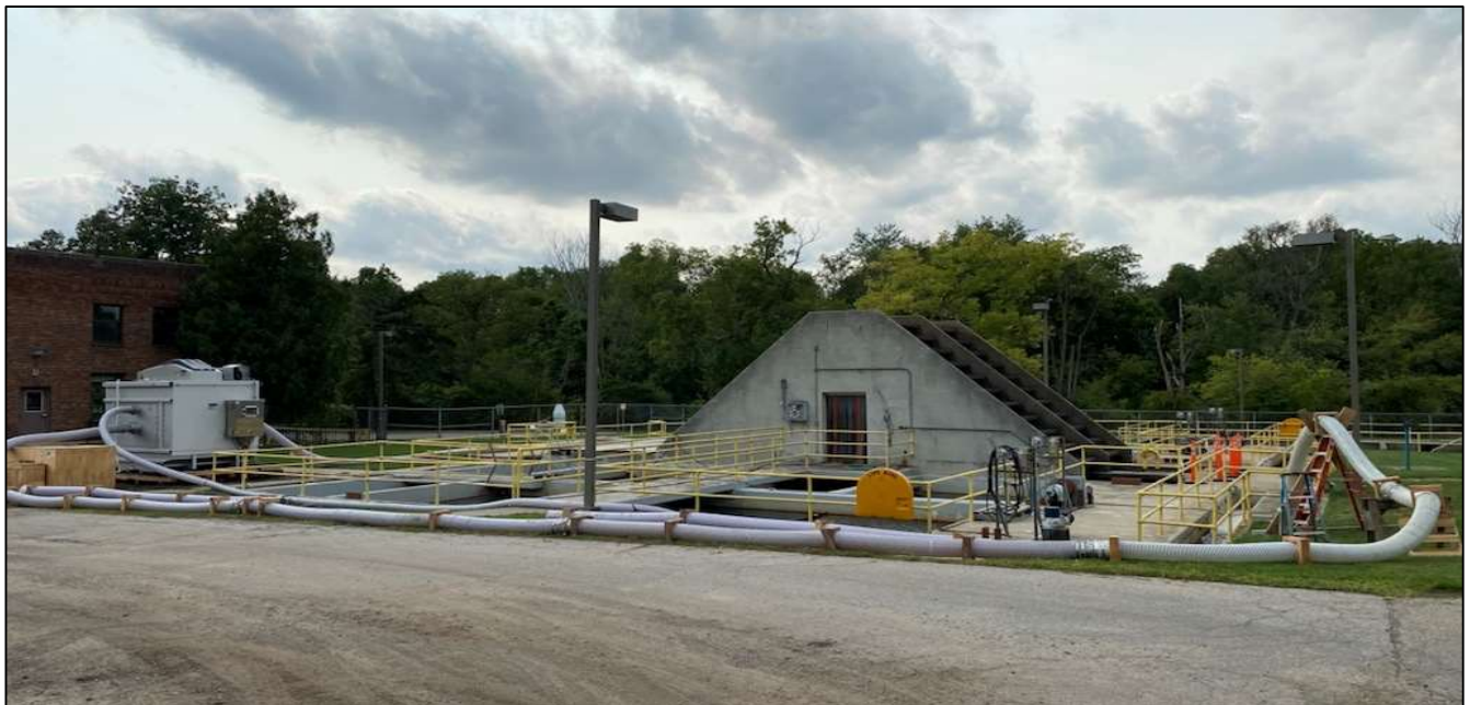
Sample pilot installation showing piping
