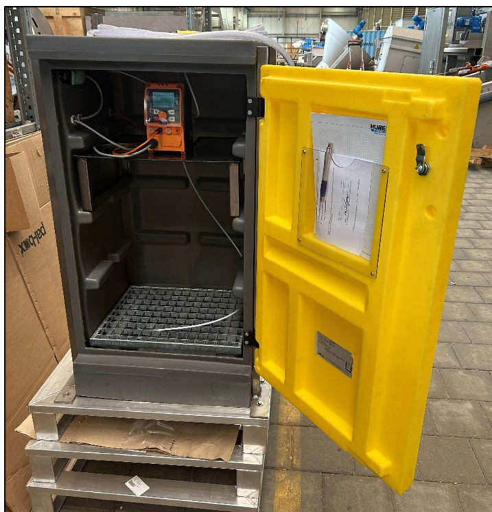
Chemical Metering Pump
