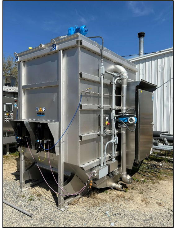
Influent & Turbidity monitoring system Control Panel
