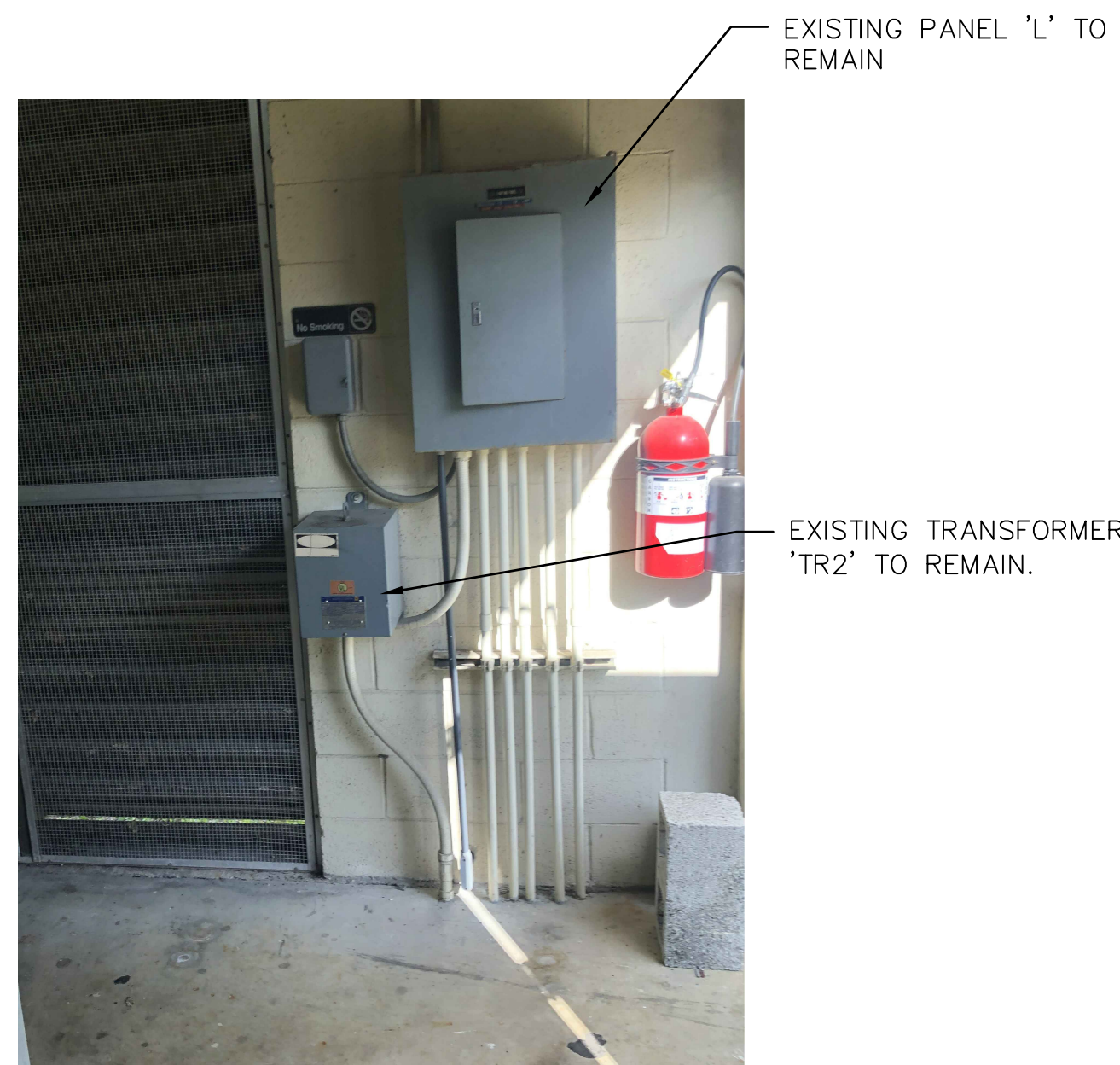
GENERATOR BUILDING PHOTO 2
