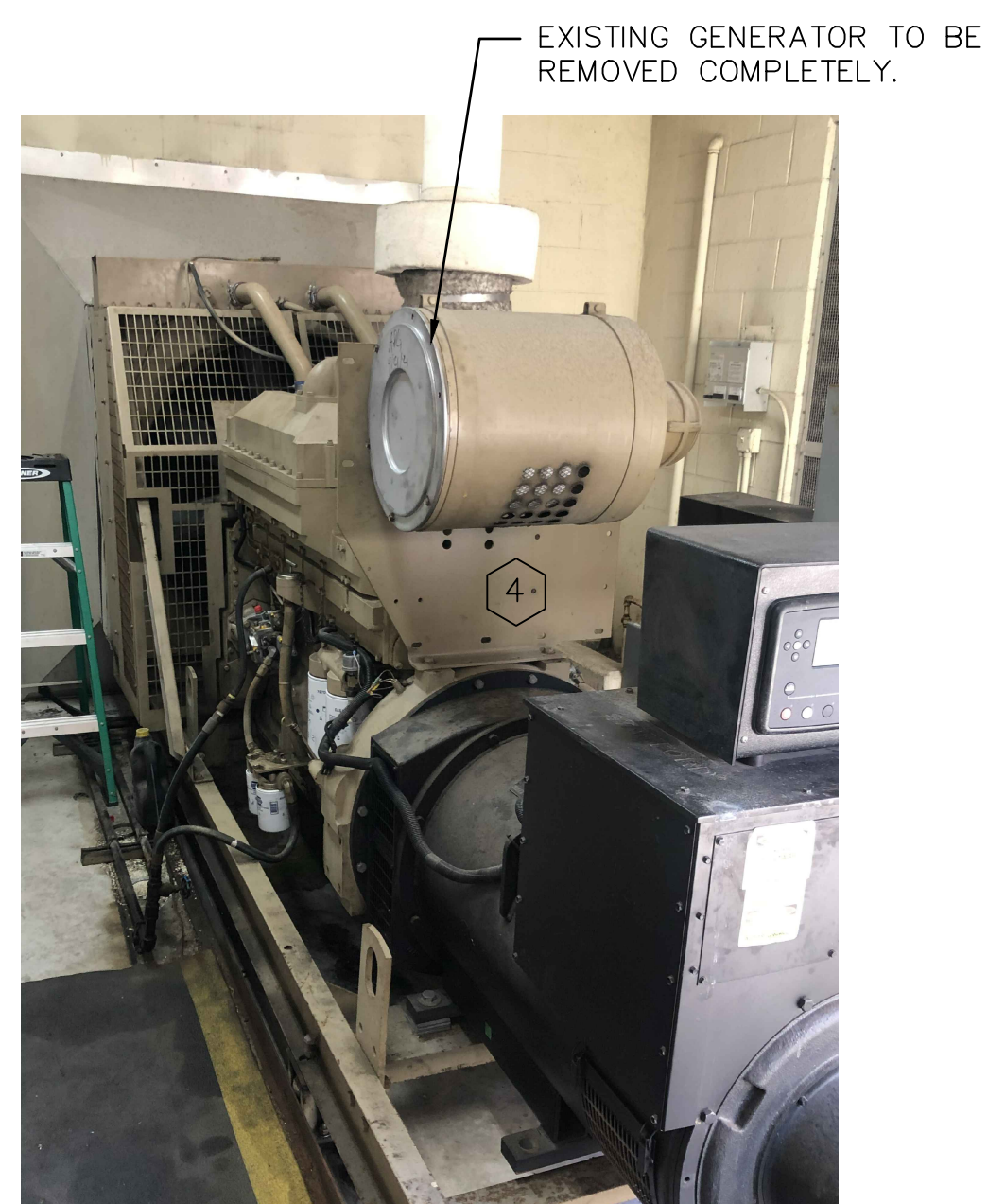
GENERATOR BUILDING PHOTO 3
