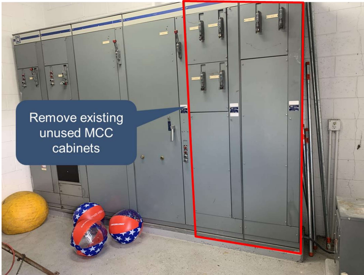
Figure 1: Photo of Existing MCCs
