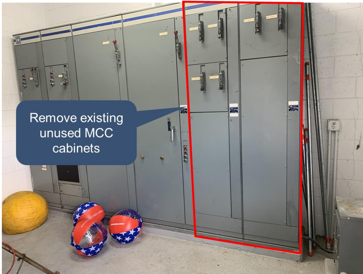
Figure 1: Photo of Existing MCCs
