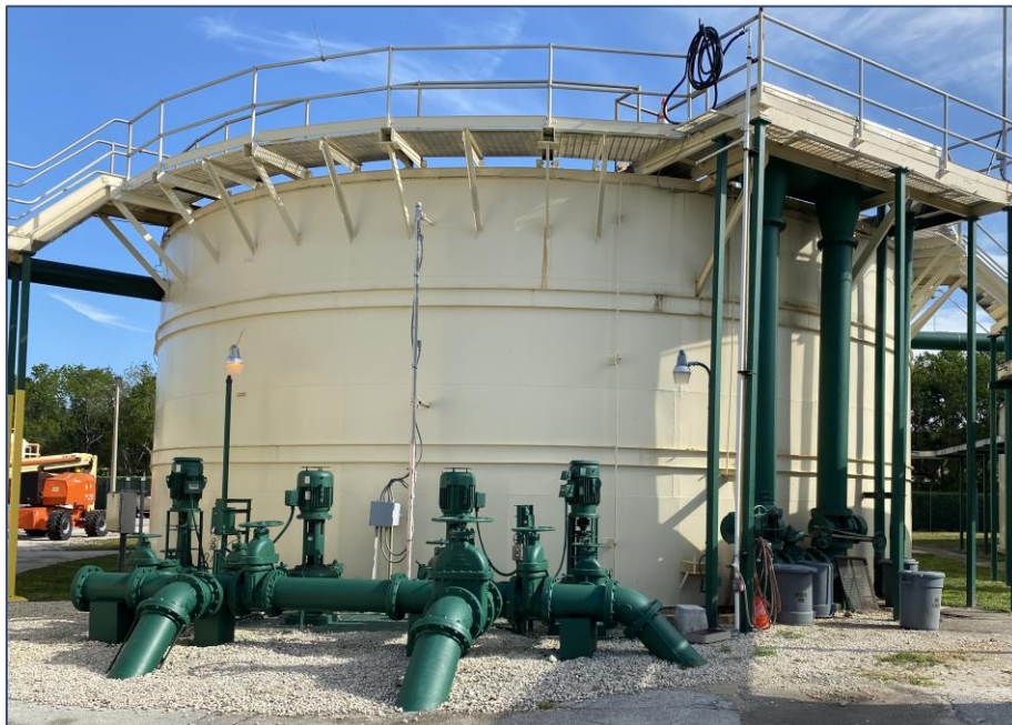
Figure 7-1: Surge Tank at the WWTP
