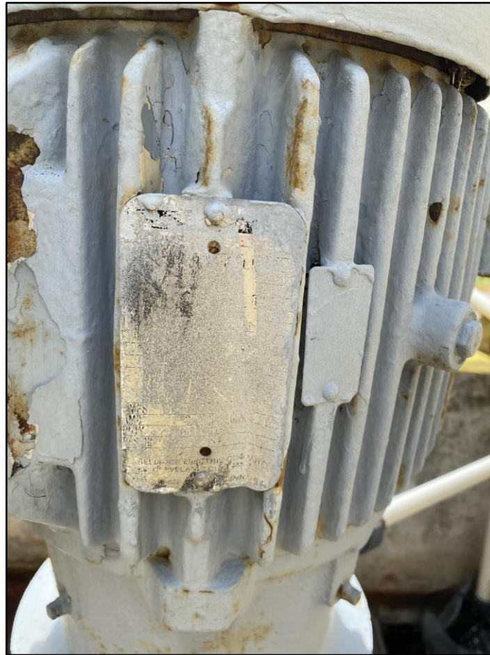
Figure 7-19: Corrosion Damage on the Digested Sludge Transfer Pump Casing
