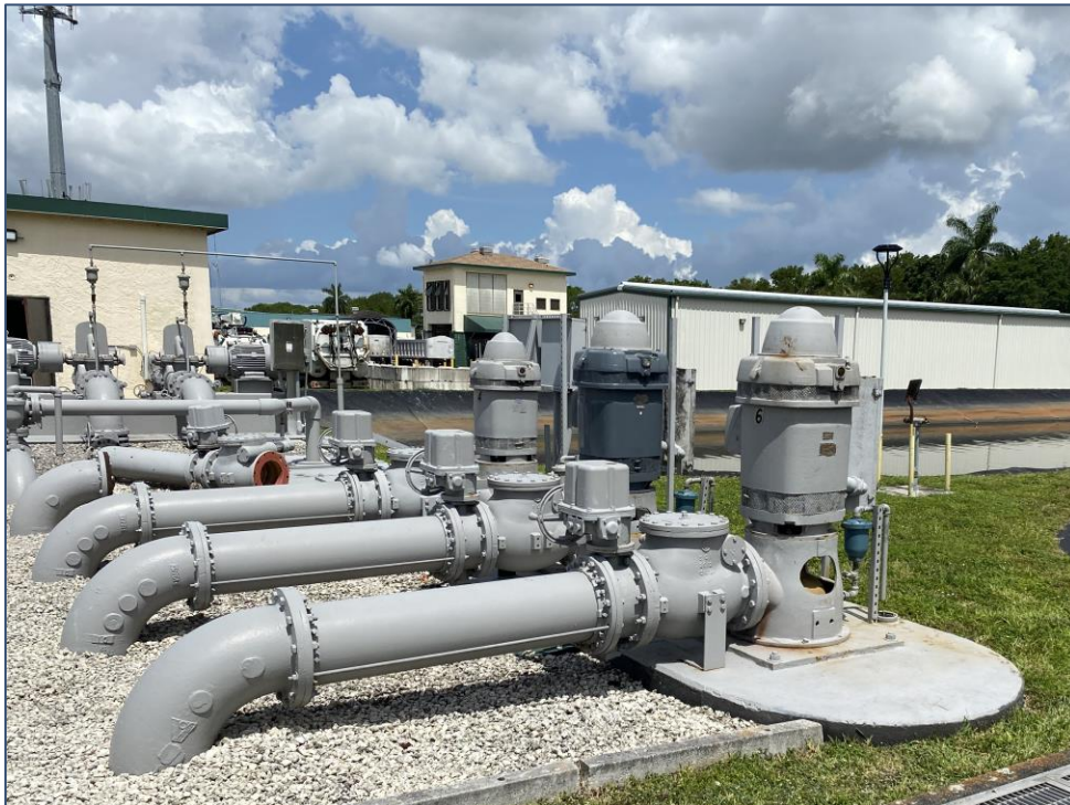
Figure 7-2: Effluent Transfer Pump Station
