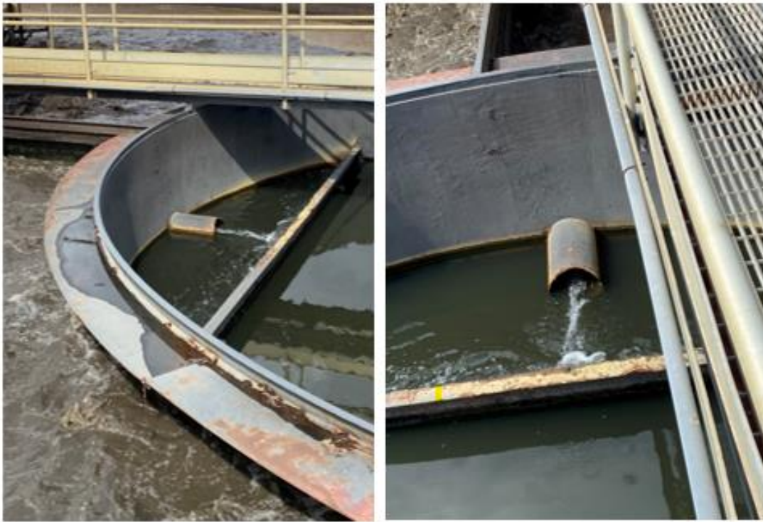
Figure 7-17: Corrosion Damage on the Secondary Effluent Transfer Line
