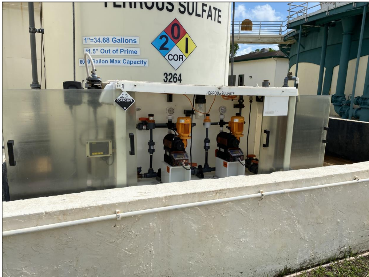
Figure 7-20: Ferrous Sulfate Dosing Skid
