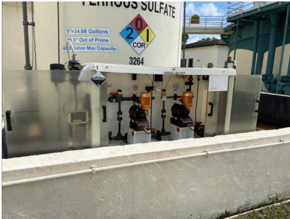
Figure 2-4: Existing Ferric/Ferrous Sulfate Dosing System
