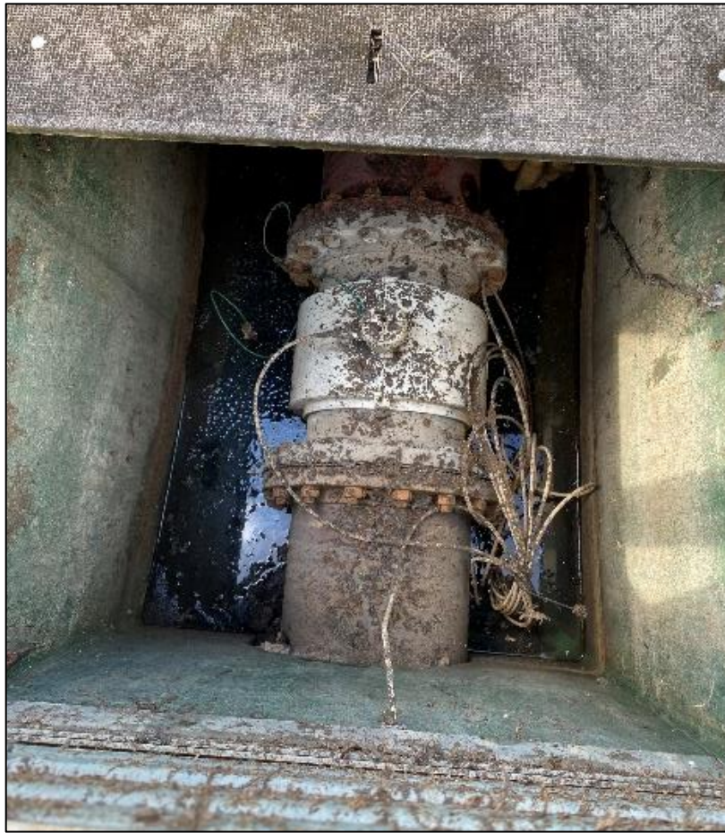
Figure 7-12: Ultrasonic Flow Meter in the Influent Transfer Line
