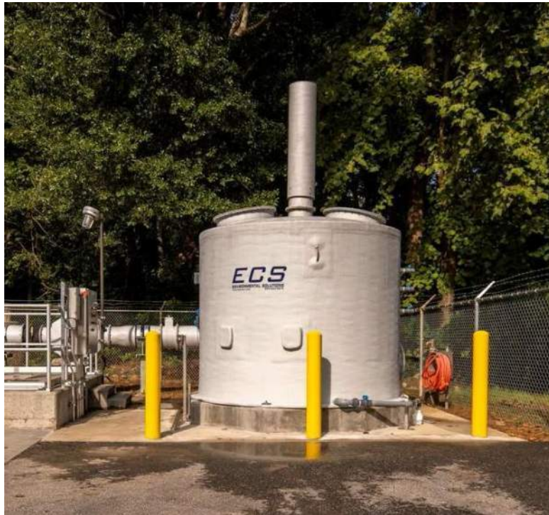
Figure 6-4: Dry Media Adsorption Deep Bed Unit
