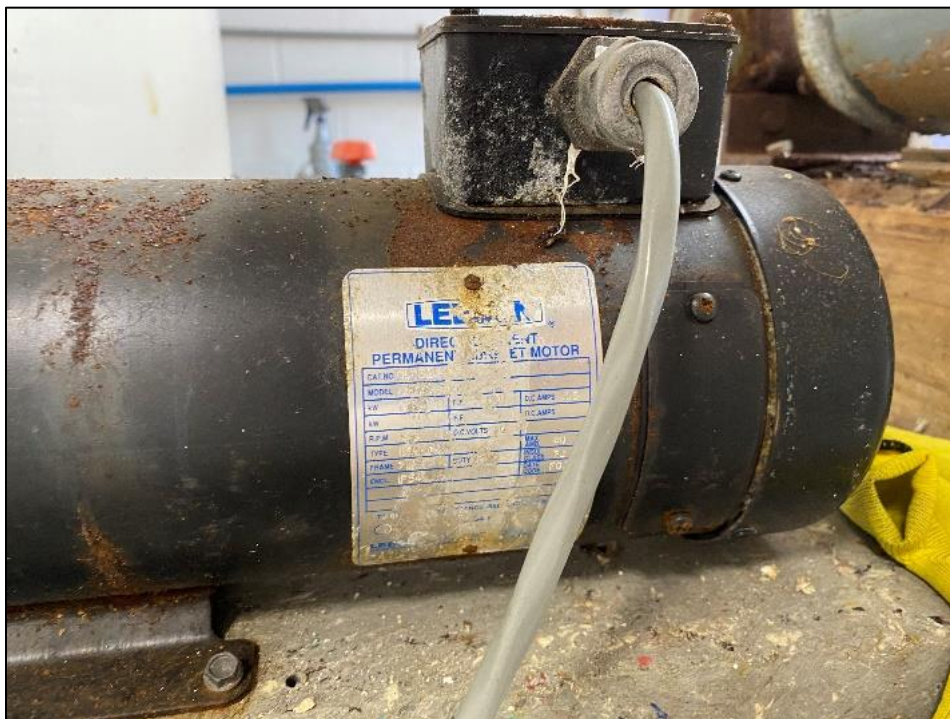
Figure 7-21: Corrosion Damage on a Polymer Transfer Pump
