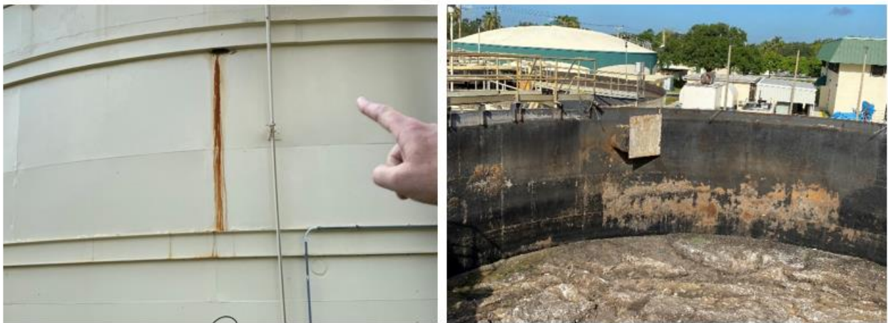
Figure 7-13: Corrosion Damage on the Surge Tank
