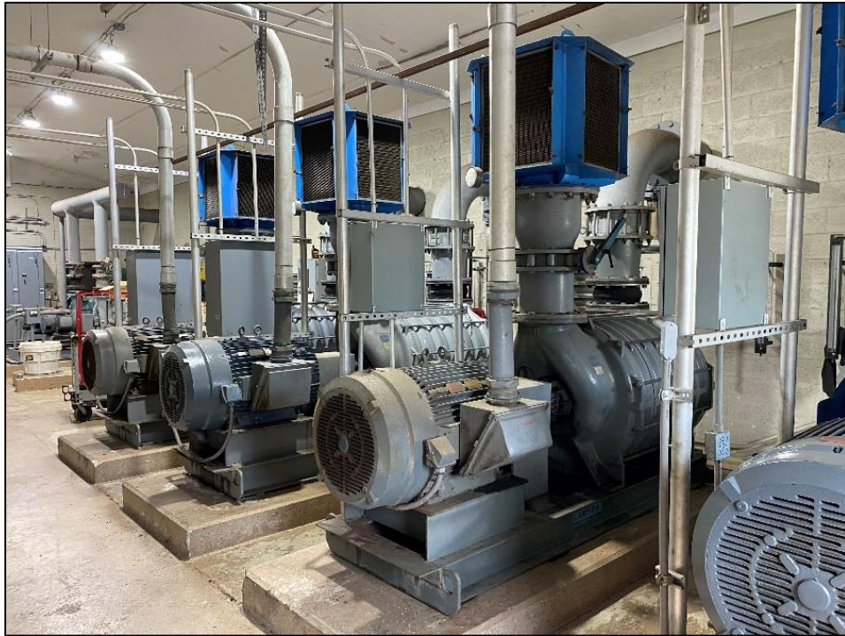
Figure 7-18: Multistage Centrifugal Blowers Used in the Cooper City WWTP
