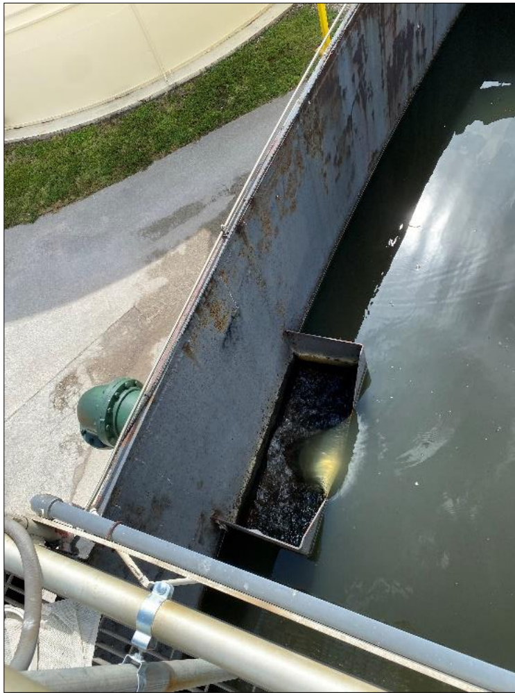
Figure 7-16: Corrosion Damage on the Package Plant 2 Wall
