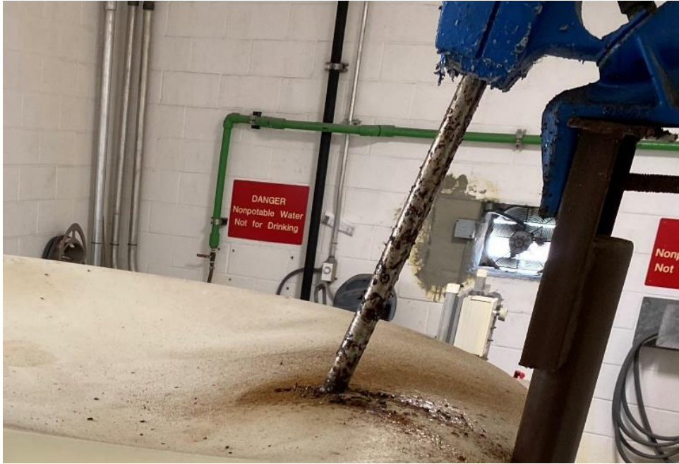
Figure 7-22: Corrosion Damage on Polymer Mixer Shaft
