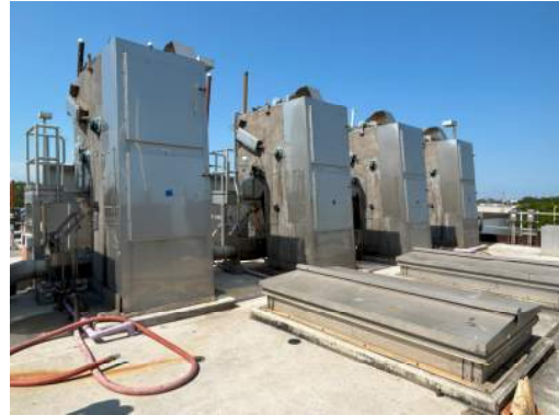
Installation of Parkson AquaGuard at Broward County NRWTP
