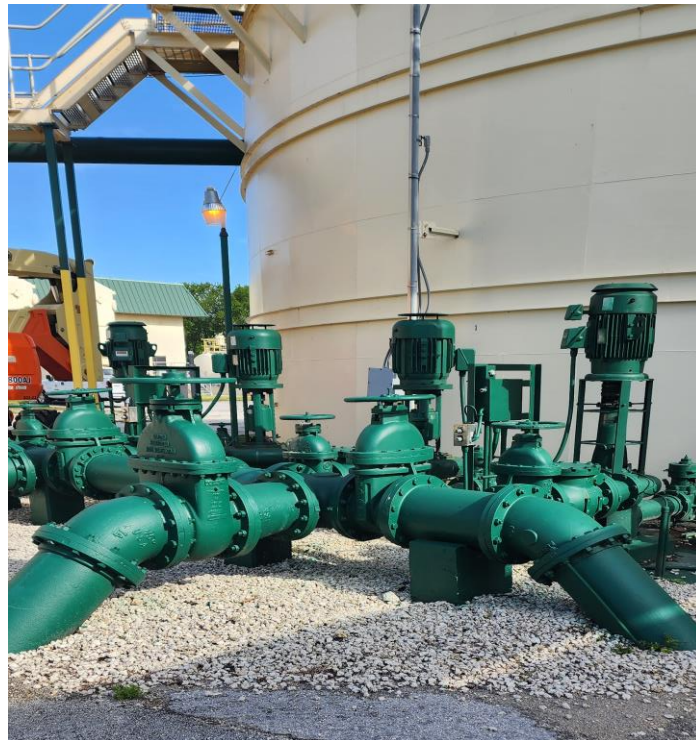
Figure 7-14: Transfer Pump Station
