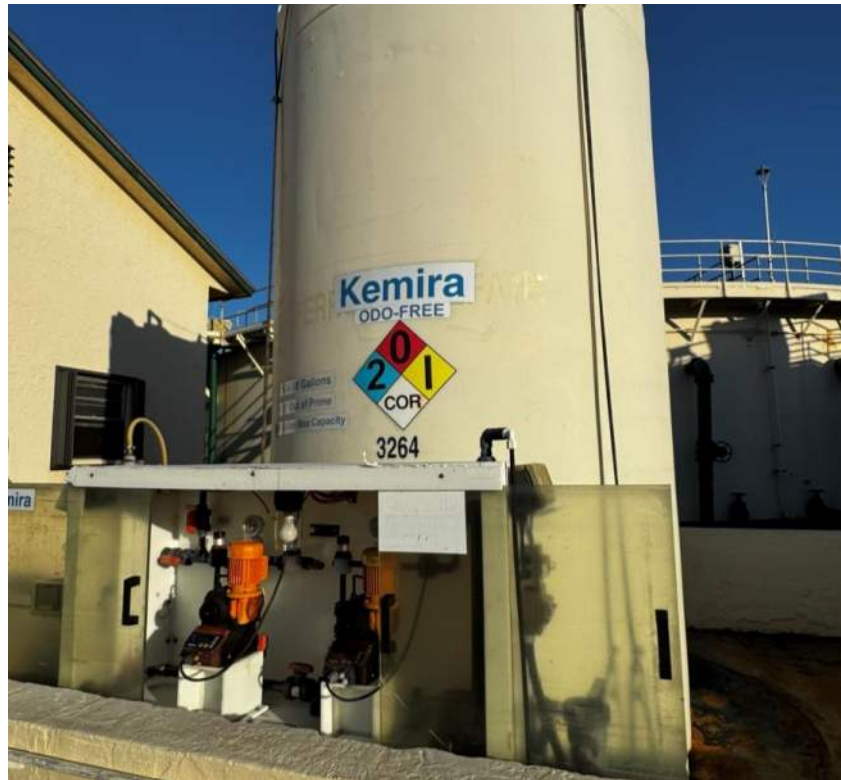
Figure 6-1: Ferric/Ferrous Sulfate Dosing System
