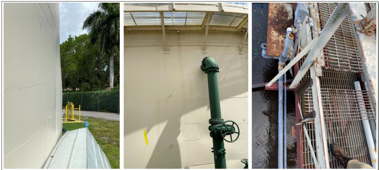
Figure 7-15: Package Plant 1 Tank Bowing/Bulging and Corrosion Damage
