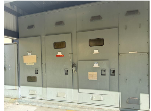
Figure 5.1. George A. Haughney Plant 23 kV main and generator power breakers refurbishment in the existing 23 kV main distribution switchgear
