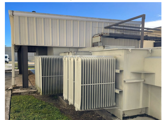
Figure 5.2. George A. Haughney Plant Transformers
