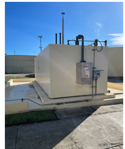
Figure 5.4. George A. Haughney Plant Diesel Fuel Tank
