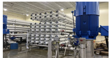
Figure 6.4. Phase III – Membrane WTP
