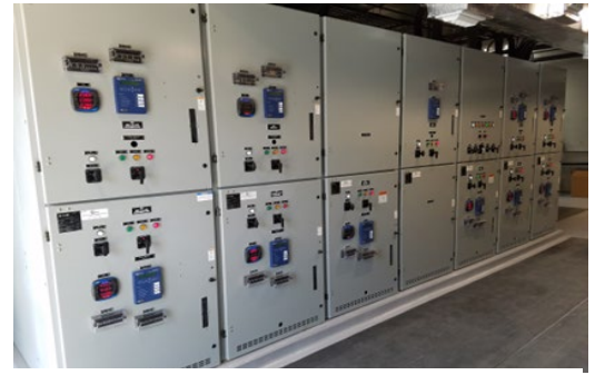
Figure 6.2. MCC in Generator Building at GTL WWTP
