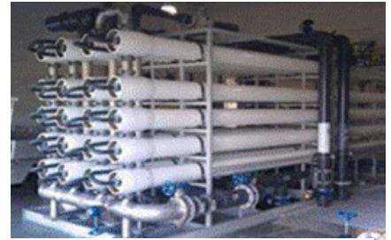
Figure 6.5. Phase II – Membrane WTP
