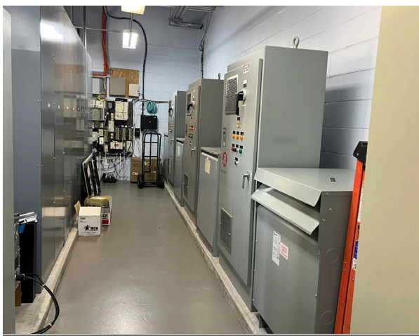
Membrane Building Electrical Room
