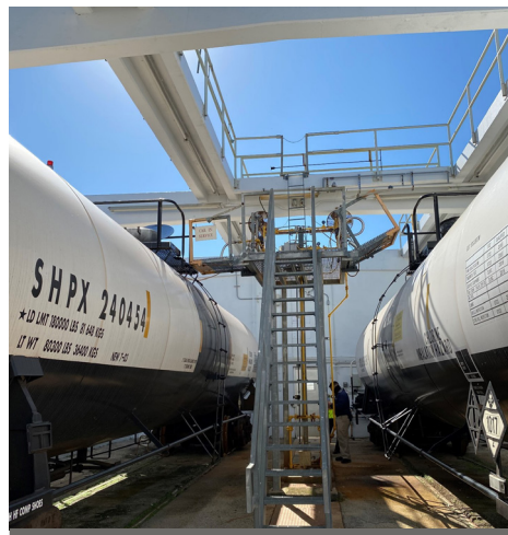
Railcar Receiving Station
