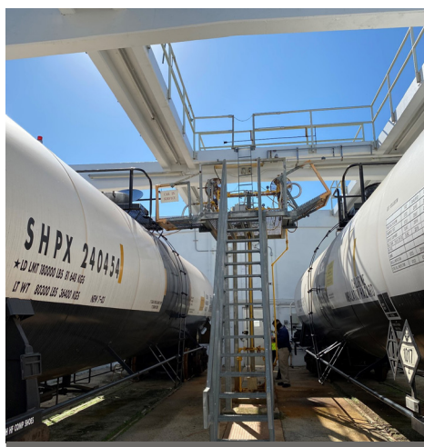
Railcar Receiving Station
