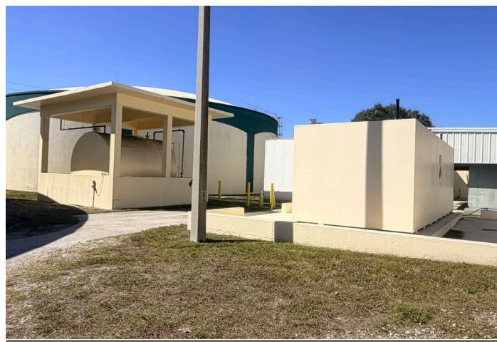
Generator in Walk-in Enclosure
