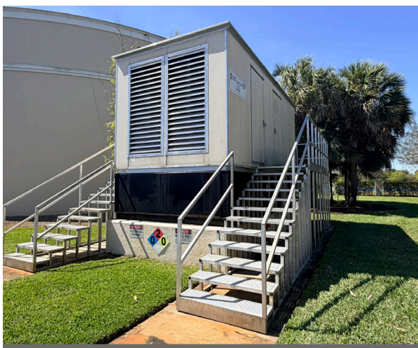
Pine Island Road Storage Pump Station - Generator
