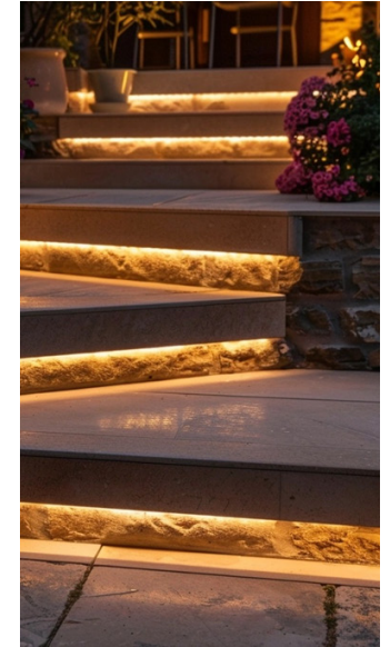
Lighting for Levee Trail stairs
