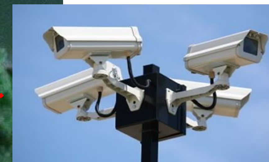
Typical Camera on on Light Posts
