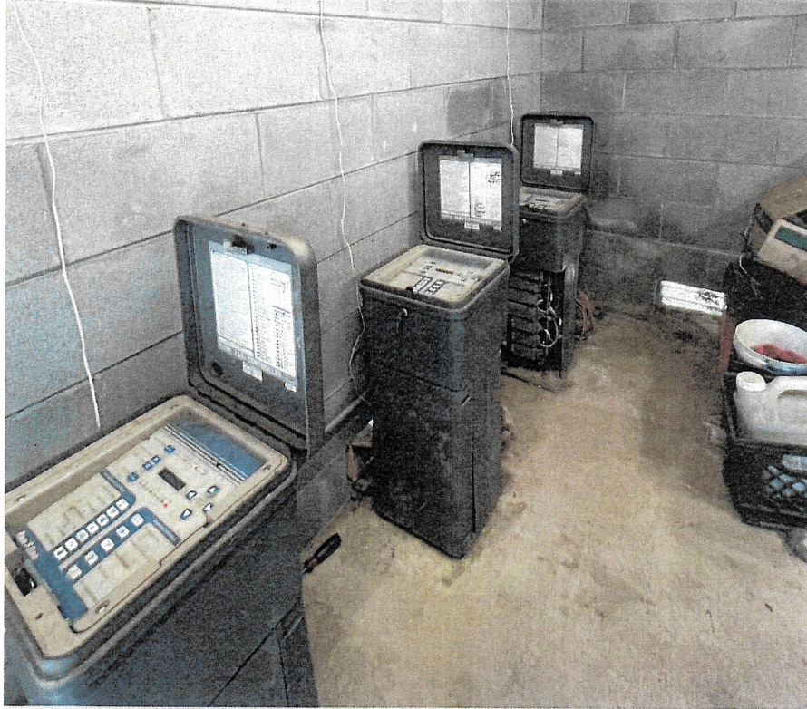
Irrigation controllers located in pumphouse.
