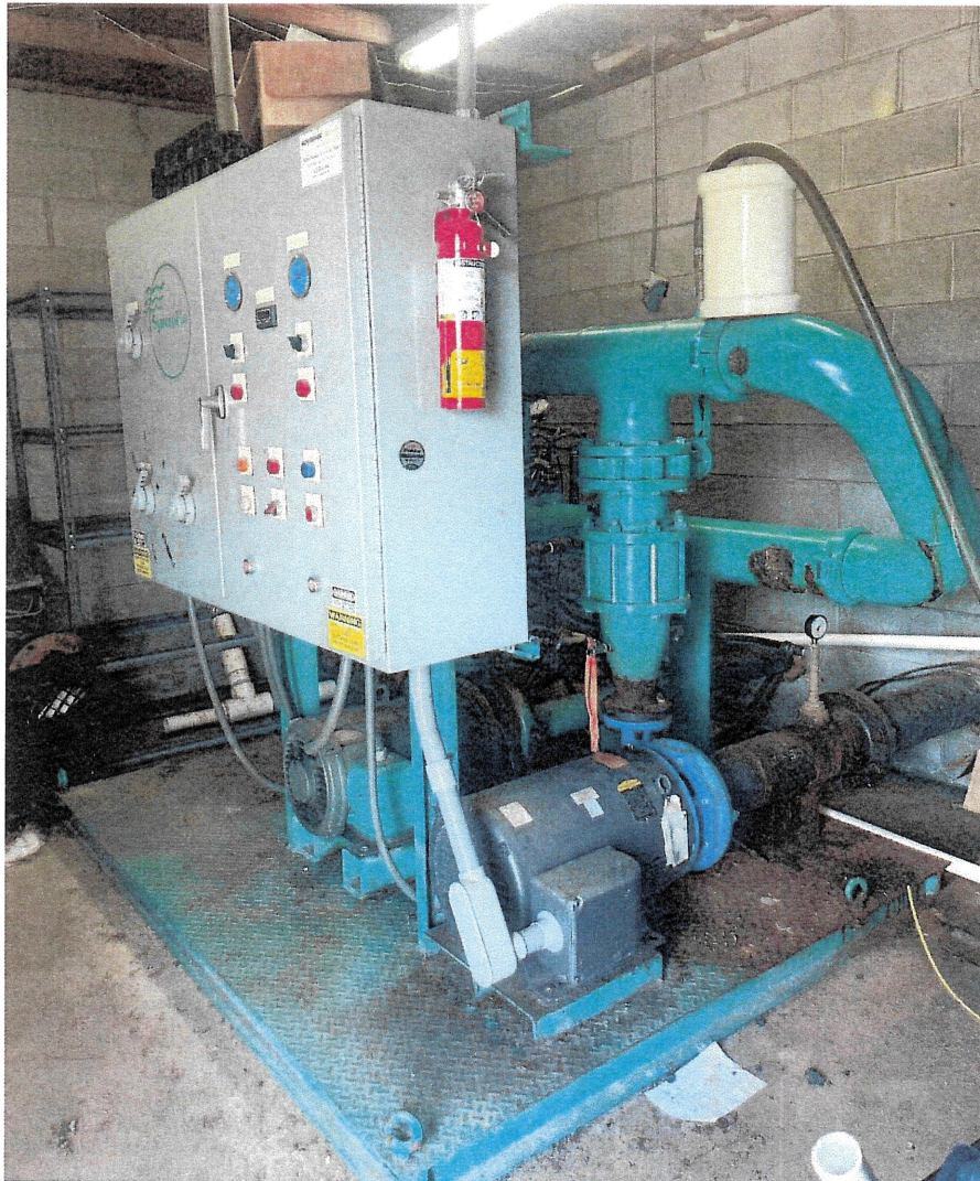
Present pump system that is showing signs of wear and tear.
