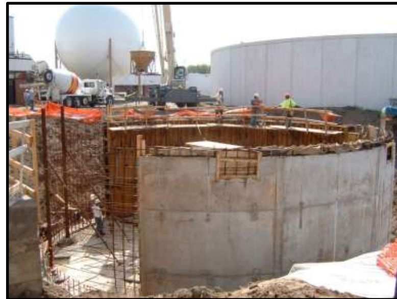
Below grade 170k gal. Receiving Tank ~2007
