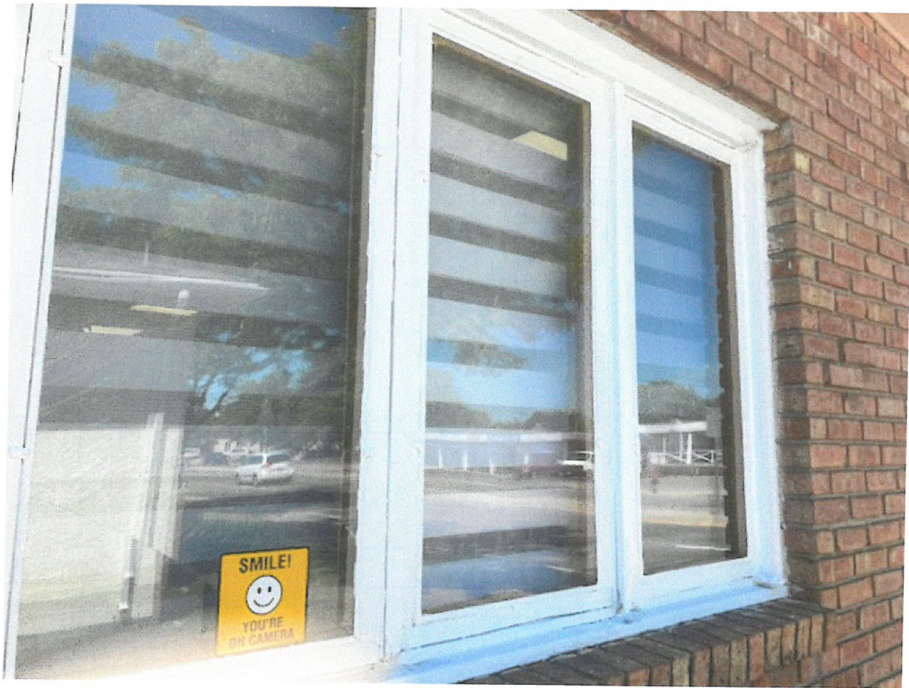
North side window (cracked, rotting)
