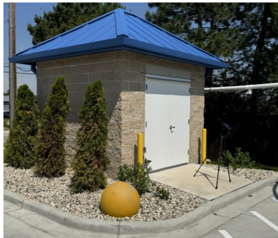
Figure 6: Vacuum Pump House
